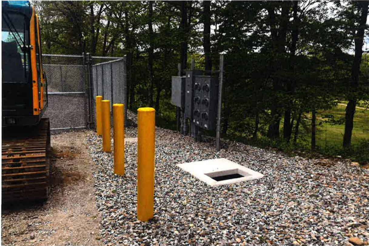
Photo 3: View of electrical board.
