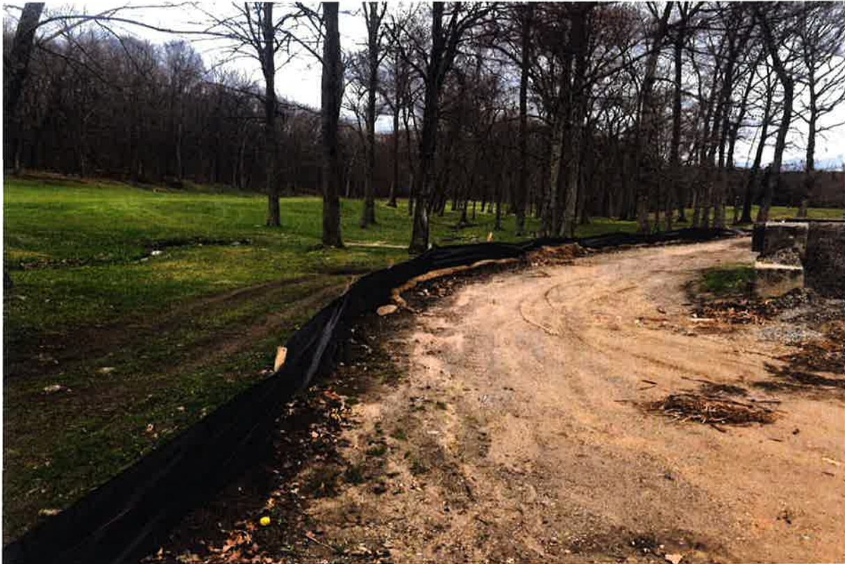
Photo 5: View of E&S perimeter controls.
