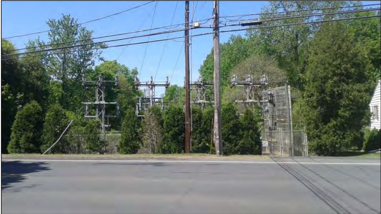
Photo 51. Overview photo of proposed project corridor facing west along an existing transmission line corridor.
