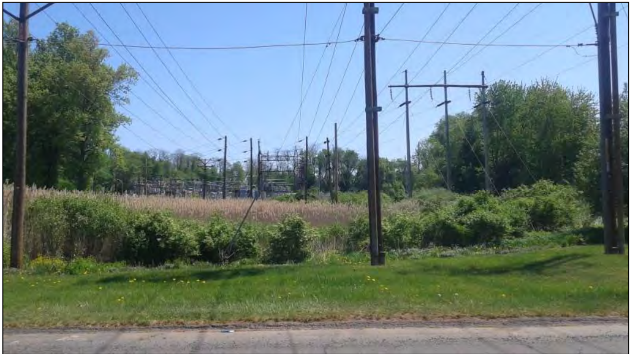
Photo 47. Overview photo of the Newington Substation facing east.
