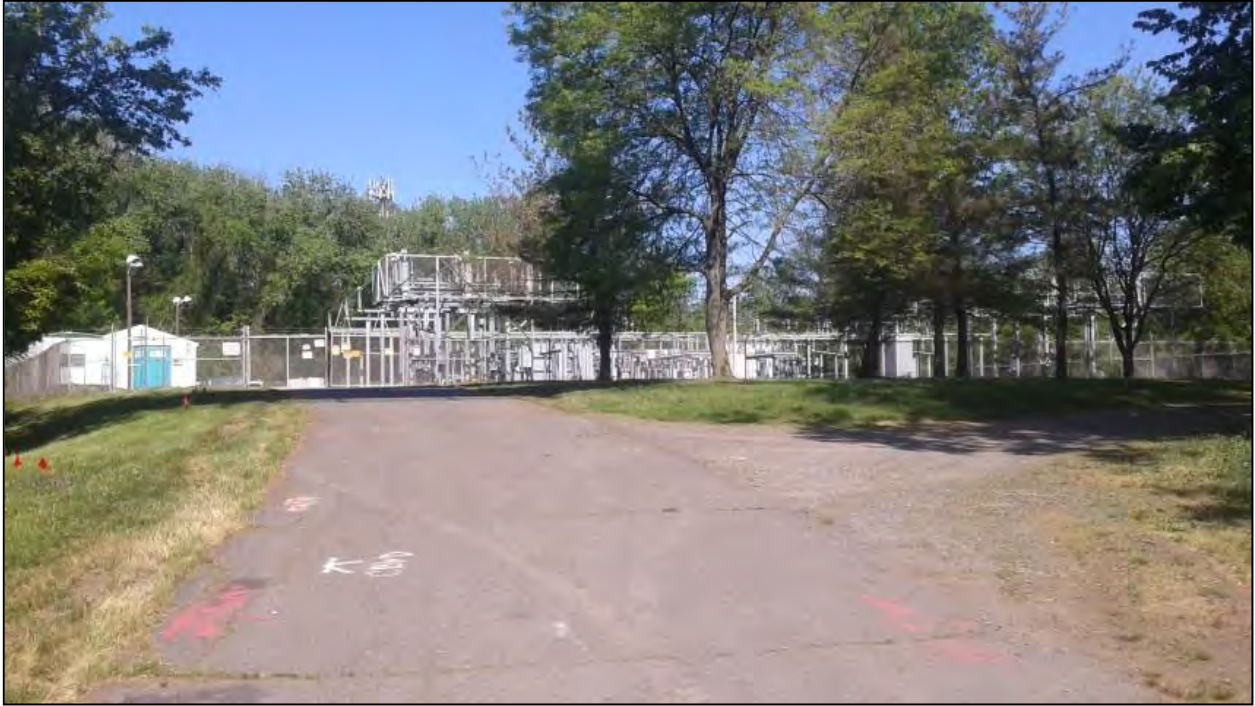
Photo 1. Overview photo of the Southwest Hartford Substation facing northwest.
