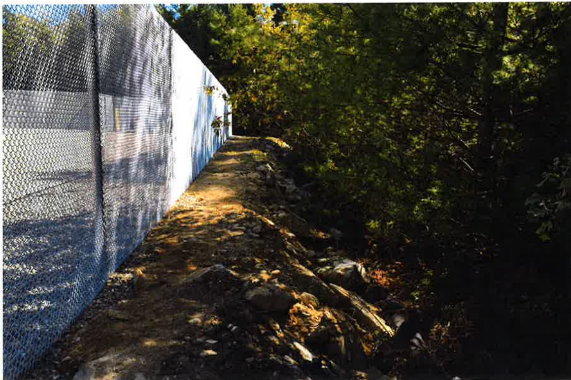
Photo 6: View of west side of compound looking south. Compost filter sock to remain in place until exposed soils are permanently stabilized with seeded vegetation.
