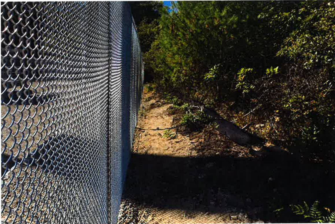
Photo 5: View of north side of compound looking west. Compost filter sock to remain in place until exposed soils are permanently stabilized with seeded vegetation.
