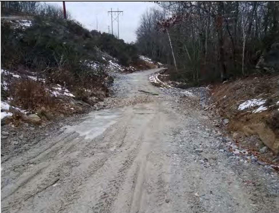
Photo 4: 12/22/2017, Watertown: Map14, CORRECTIVE ACTION- Access road between Str38 and Str39 graded, water bar and drainage swale reformed.
