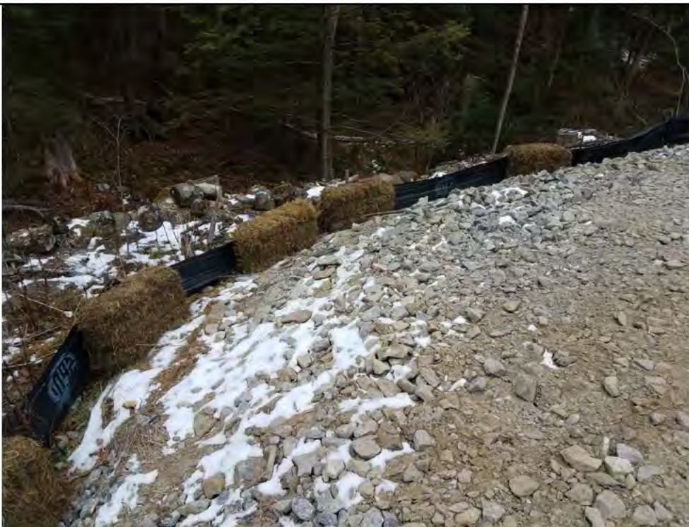
Photo 8: 12/22/2017, Harwinton: Map 32, CORRECTIVE ACTION - At edge of Str87 pad and S-F11/S-F10/W-F11, repaired silt fence and added hay bales.
