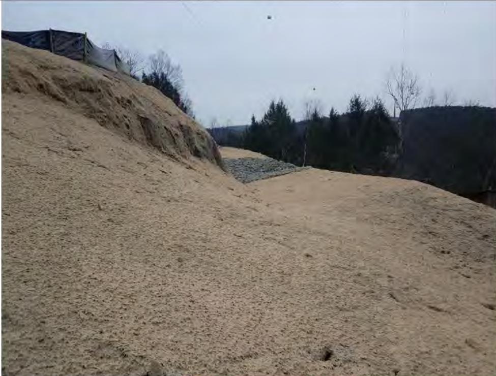
Photo 13: 12/22/2017, Litchfield: Str86, Str3236, and Str3171, restoration of slope and pad surfaces, area stabilized with hydroseed.
