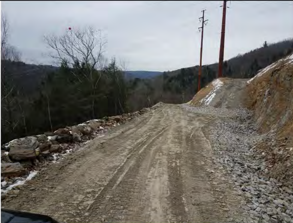
Photo 11: 12/22/2017, Litchfield: Access road to Str86, Str3236, and Str3171, graded, and stone filled drainage swale.
