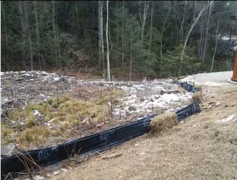
Photo 7: 12/22/2017, Harwinton: Map 32, CORRECTIVE ACTION - At edge of Str87 pad and W-F12/S-F11, repaired silt fence and added hay bales.
