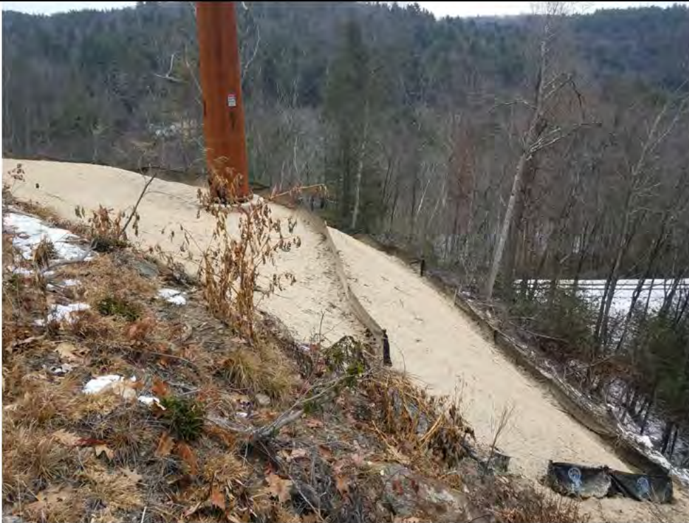
Photo 14: 12/22/2017, Litchfield: Str86, Str3236, and Str3171, restoration of slope and pad surfaces, area stabilized with hydroseed, installation of silt fence.
