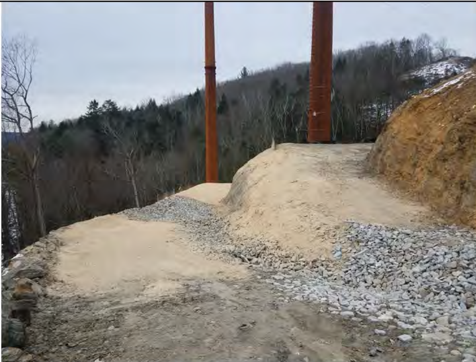
Photo 12: 12/22/2017, Litchfield: Access road to Str86, Str3236, and Str3171, restoration of slope and pad surfaces, area stabilized with hydroseed, stone filled drainage swale.
