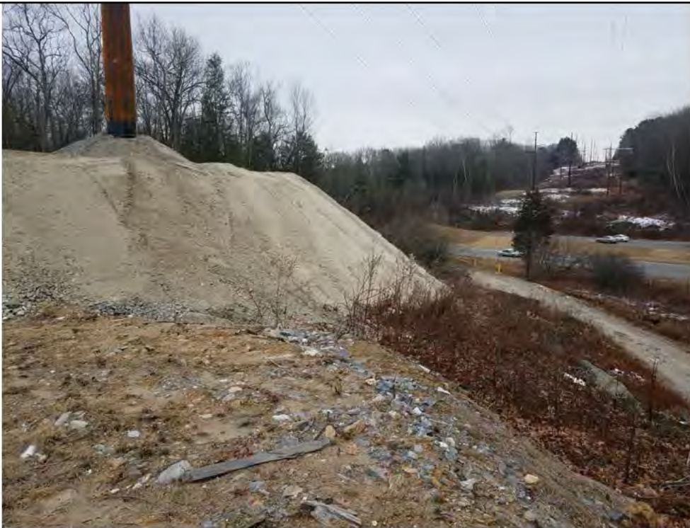
Photo 10: 12/22/2017, Litchfield: Map 30, Str85, restoration started, slope stabilization required.
