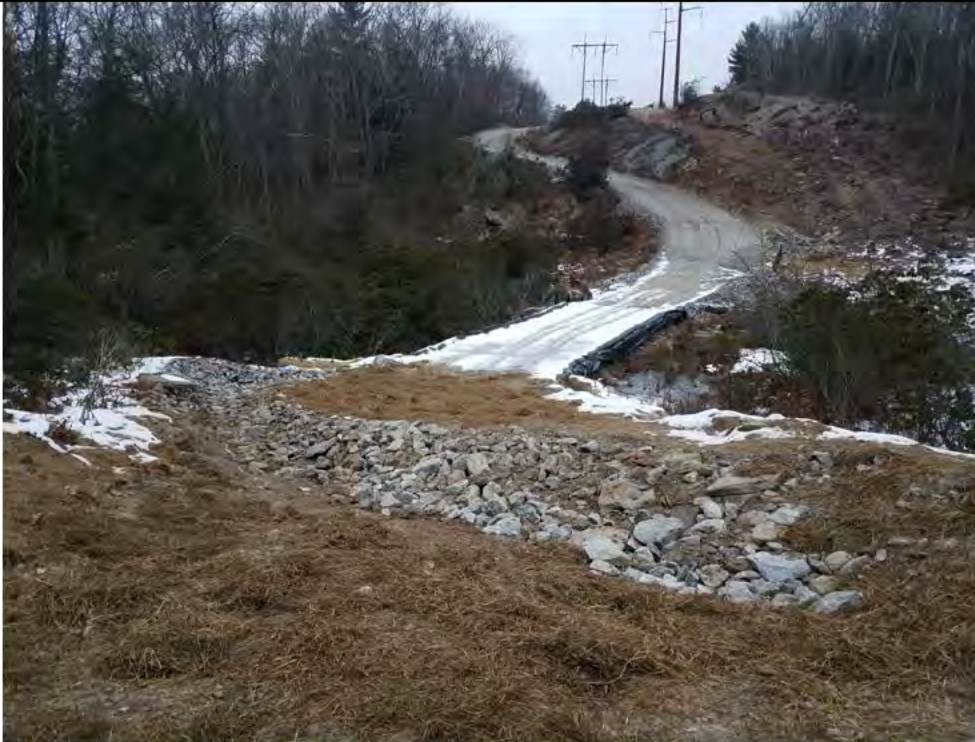
Photo 2: 12/22/2017, Watertown: Map14, CORRECTIVE ACTION- Upland of W-C20/VP-C20-1, access road grading, construction of stone filled water bar, and straw mulch for stabilization.
