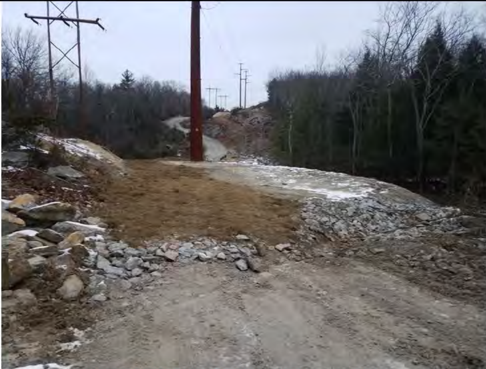
Photo 3: 12/22/2017, Watertown: Map14, CORRECTIVE ACTION-Str39 pad, graded pad, added straw mulch for stabilization, reformed water bar, lined water bar with stone.
