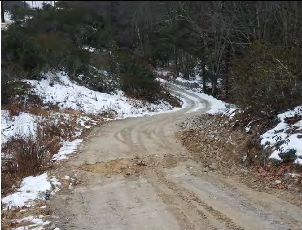
Photo 5: 12/22/2017, Watertown: Map12, CORRECTIVE ACTION- Access road between Str34 and Str35, graded access road, reformed water bar, and cleaned drainage swale.
