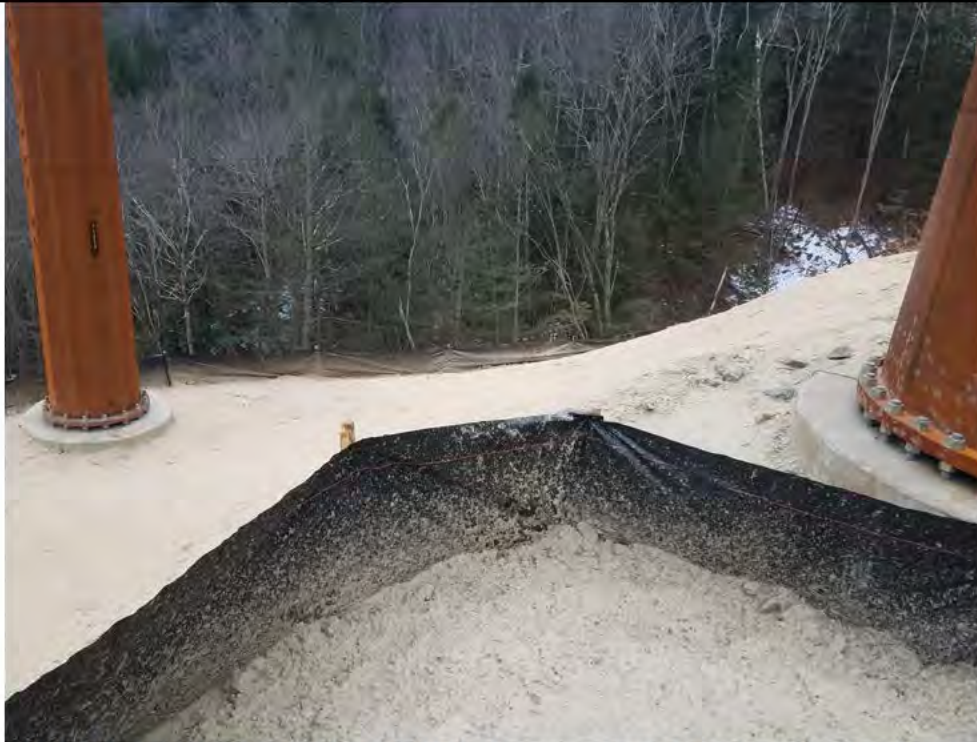
Photo 15: 12/22/2017, Litchfield: Str86, Str3236, and Str3171, restoration of slope and pad surfaces, area stabilized with hydroseed, installation of silt fence.
