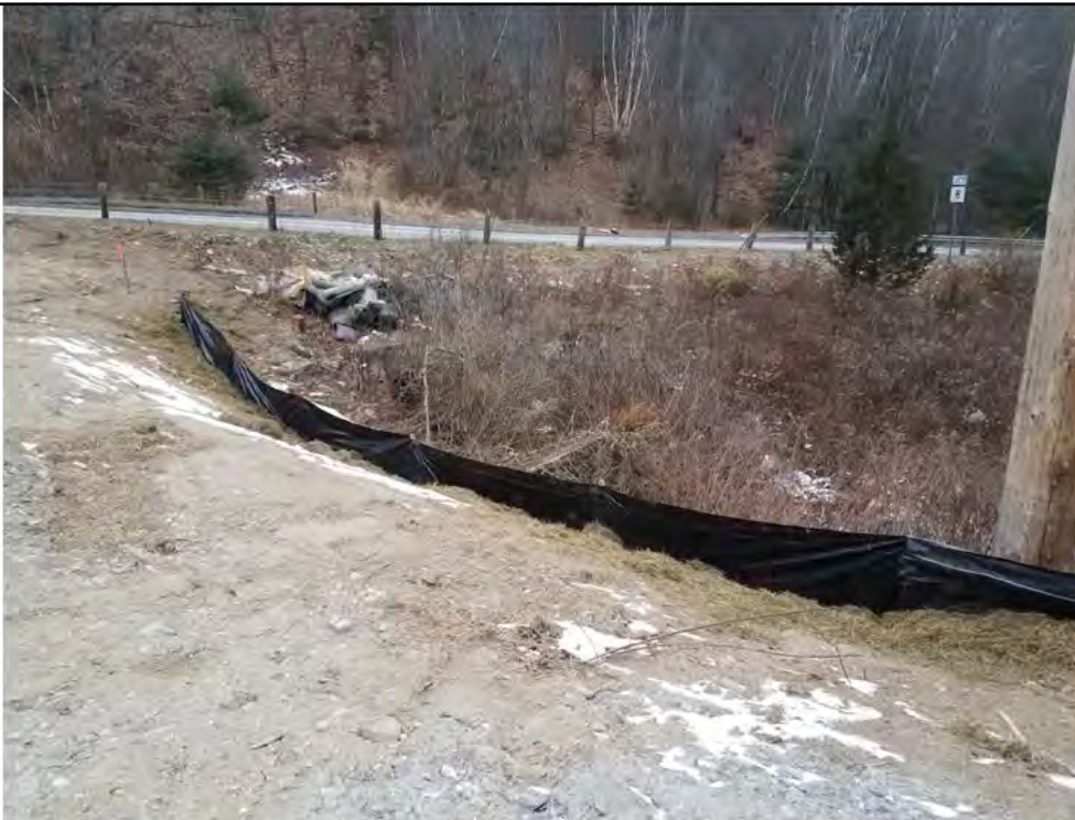
Photo 6: 12/22/2017, Watertown: Map 1, Installed silt fence at north corner of pad abutting watercourse S-A1.
