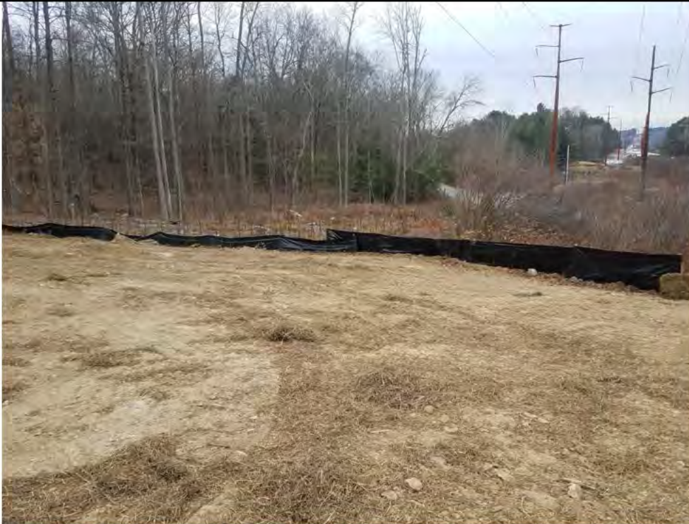
Photo 9: 12/22/2017, Harwinton: Map 35, CORRECTIVE ACTION- South edge of Str96 pad, repaired silt fence and added approximately 20' of new silt fence.
