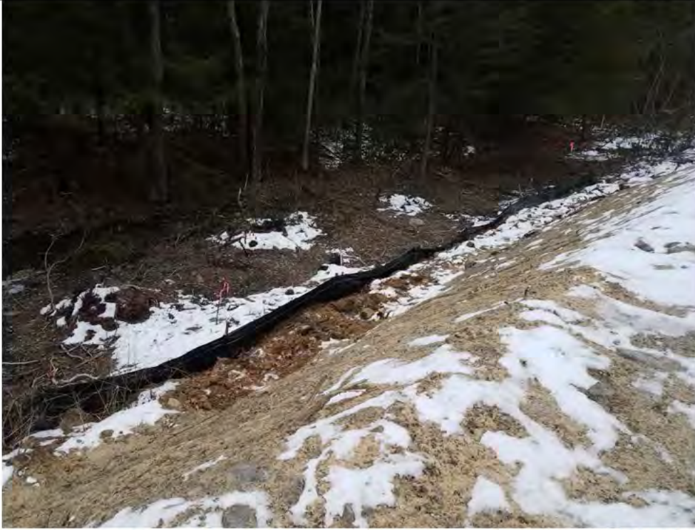
Photo 1: 12/22/2017, Watertown: Map14, CORRECTIVE ACTION- Str39, Silt fence repaired at toe of slope
