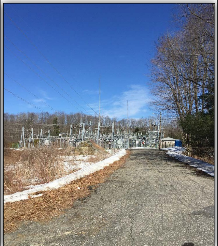
Photo 12: Campville Substation, Harwinton. View of substation, looking north from station access road off Wildcat Hill Road
