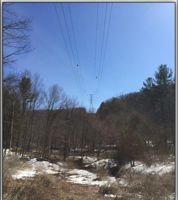
Photo 20: Valley Road, Harwinton. View to southwest of existing transmission line ROW, looking across Naugatuck River toward State Route 8.
