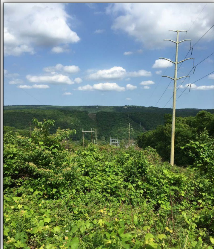
Photo 3: View of Frost Bridge Substation from Jericho Trail, Watertown. View to east along ROW from Trail crossing.
