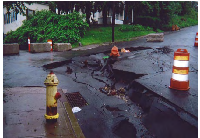
5th Street damage after storm, Waterbury
