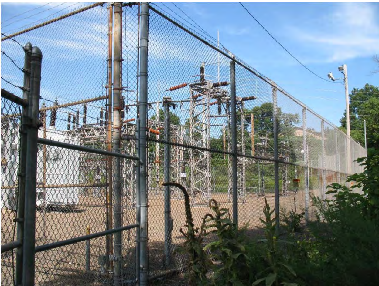
4. View west at the existing Baird Sub-station property south of the Site.
