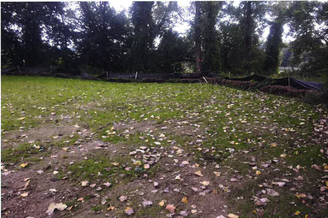
Photo 4: View of silt fence/hay bale perimeter (background) and stabilized soils (foreground) looking south.
