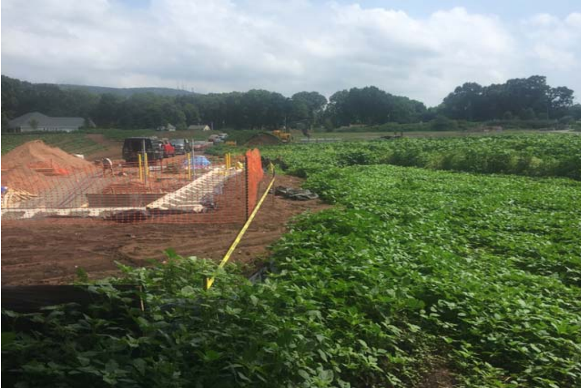
Photo 3: View of CA#2 break in silt fence requiring repair looking south; compound in left side of photo.
