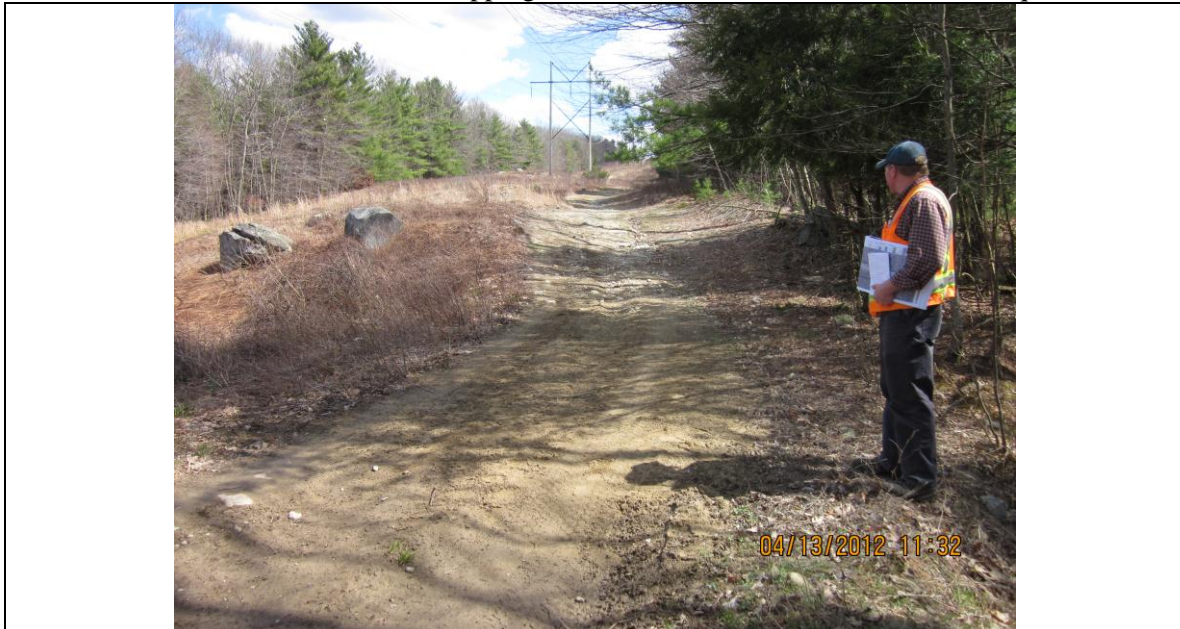
IMG_0225 Taken facing northeast at Station 1912+50 showing recent repair of access road in foreground apparently from road overtopping at blocked cross culvert. Note erosion from access road drains into wetlands/watercourses.
