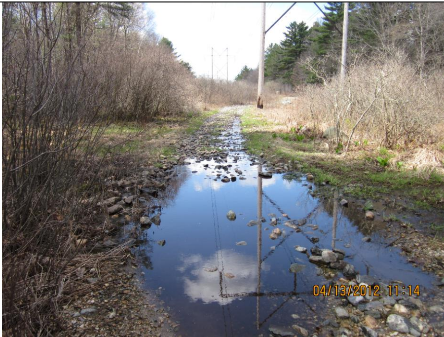
IMG_0224 Taken facing southwest at a low point in the access road showing conditions caused by a watercourse flowing down the access road.
