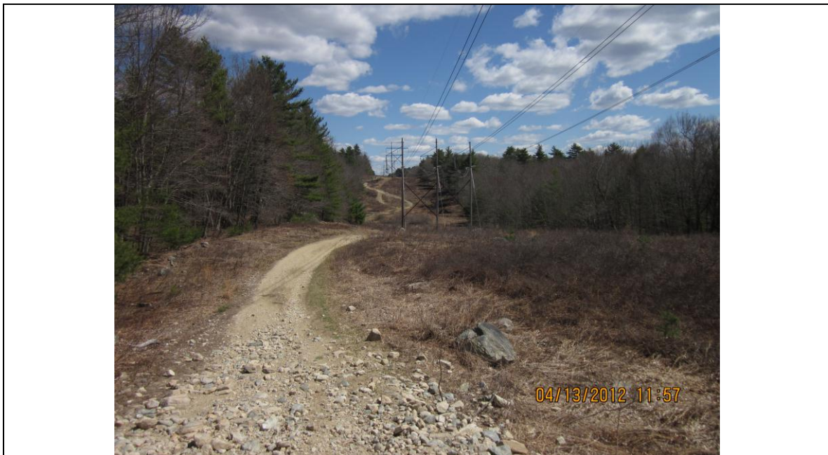
IMG_0226 Taken facing northeast at Station 1940± showing eroded steep access road and condition of access road as it approaches wetlands near the Rhode Island border.
