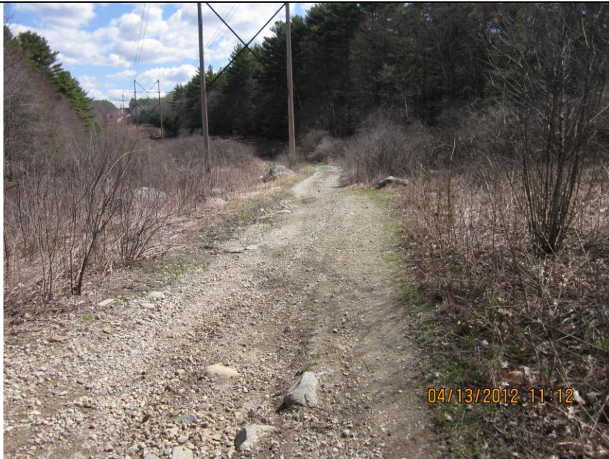
IMG_0222 Taken facing northeast just northeast of photo IMG_0223 showing continued evidence of water flow along access roadway. Note water flow exists roadway near central portion of photo. Station 1898 is in background.
