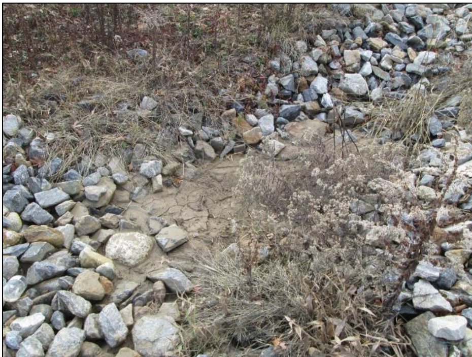
Photo #4: Sedimentation basin at Str 337. Recommend removing all accumulated sediment. (12/10)
