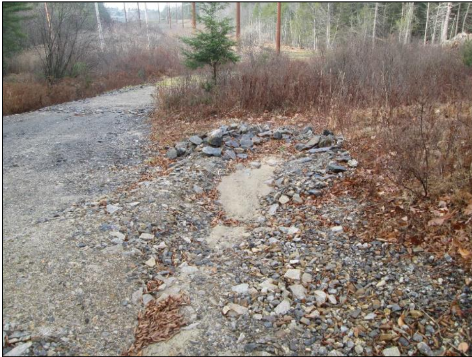
Photo #3: Sedimentation basin on access road between Str 307 and 308. Recommend removing all accumulated sediment. (12/10)
