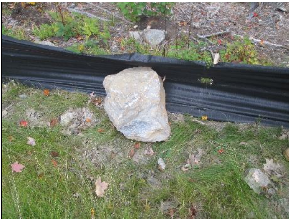
Photo #16: Silt fence torn by loose boulder. (10/9)
