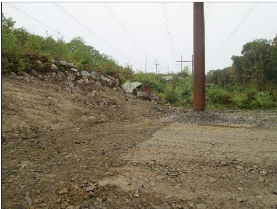
Photo #4: Re-grading and general earthwork at Str 127 as part of restoration operations. (10/2)
