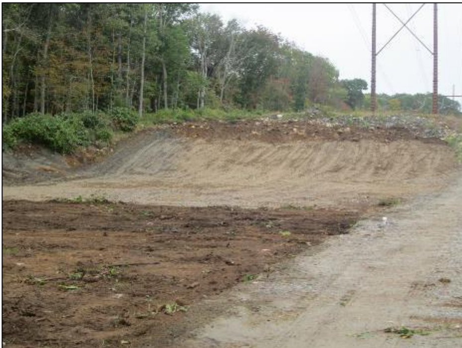
Photo #2: Re-grading and general earthwork at Str 103 as part of restoration operations. (10/2)
