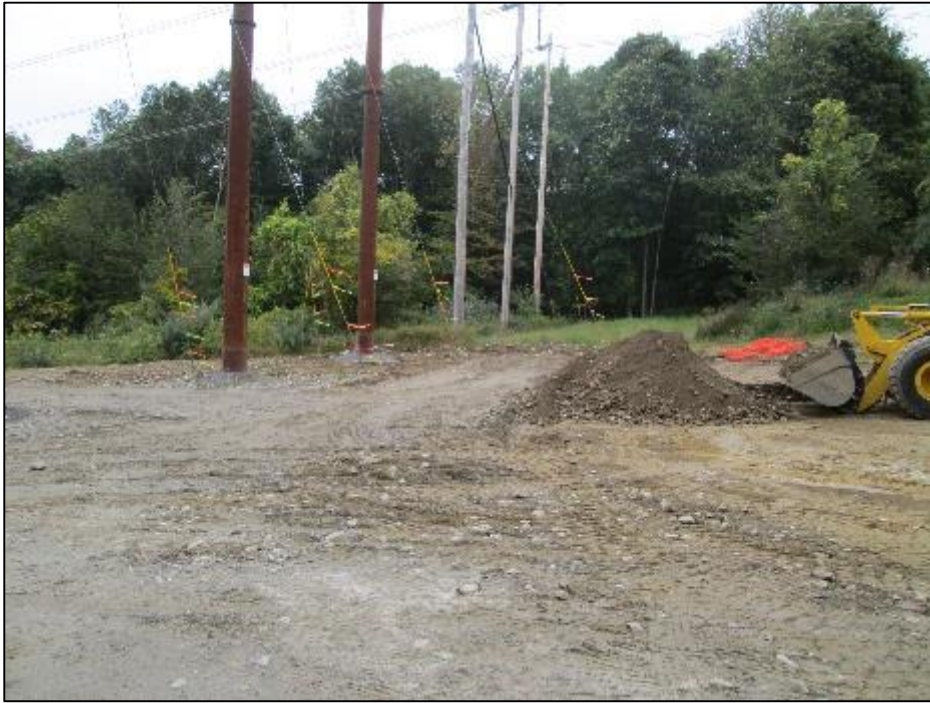
Photo #1: Re-grading and general earthwork at Str 72 as part of restoration operations. (10/2)
