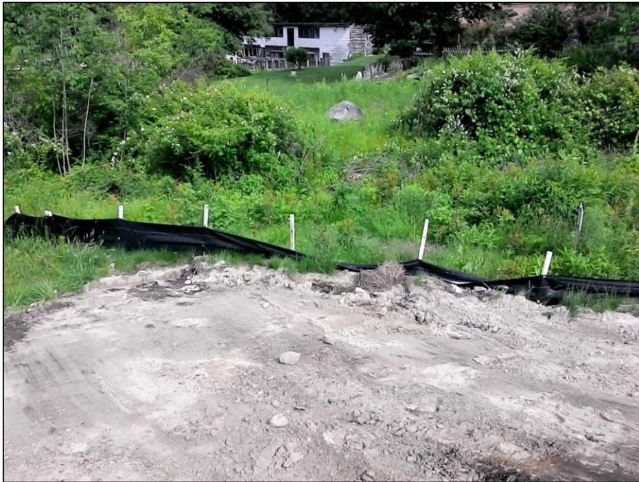
Photo #9: Area of damaged silt fence at Str 121. (6/18)
