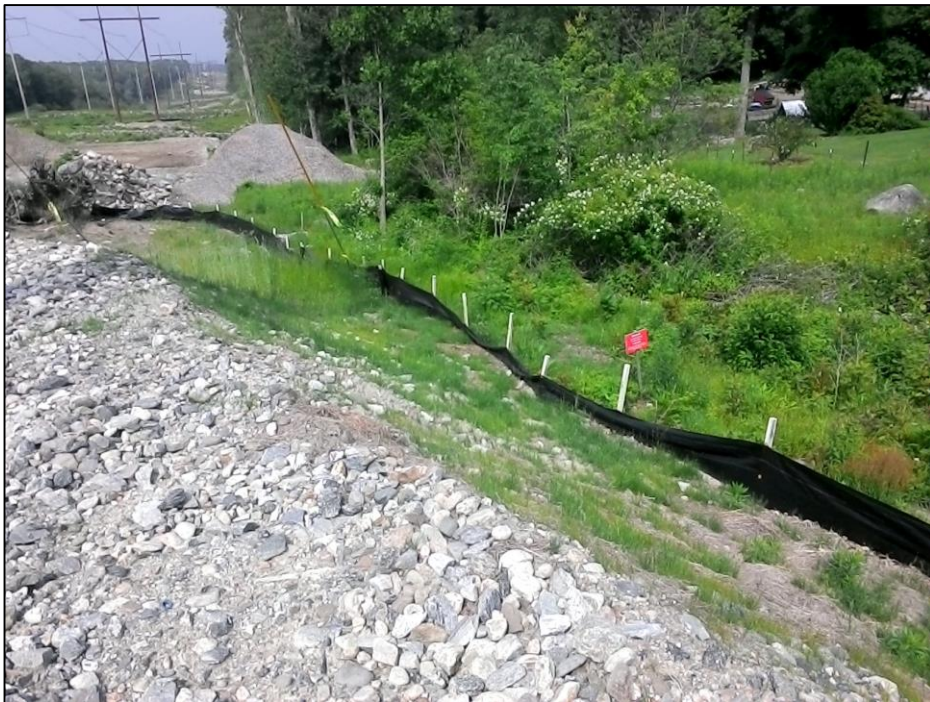
Photo #4: Area of silt fence in need of repair at Str 121. (6/11)
