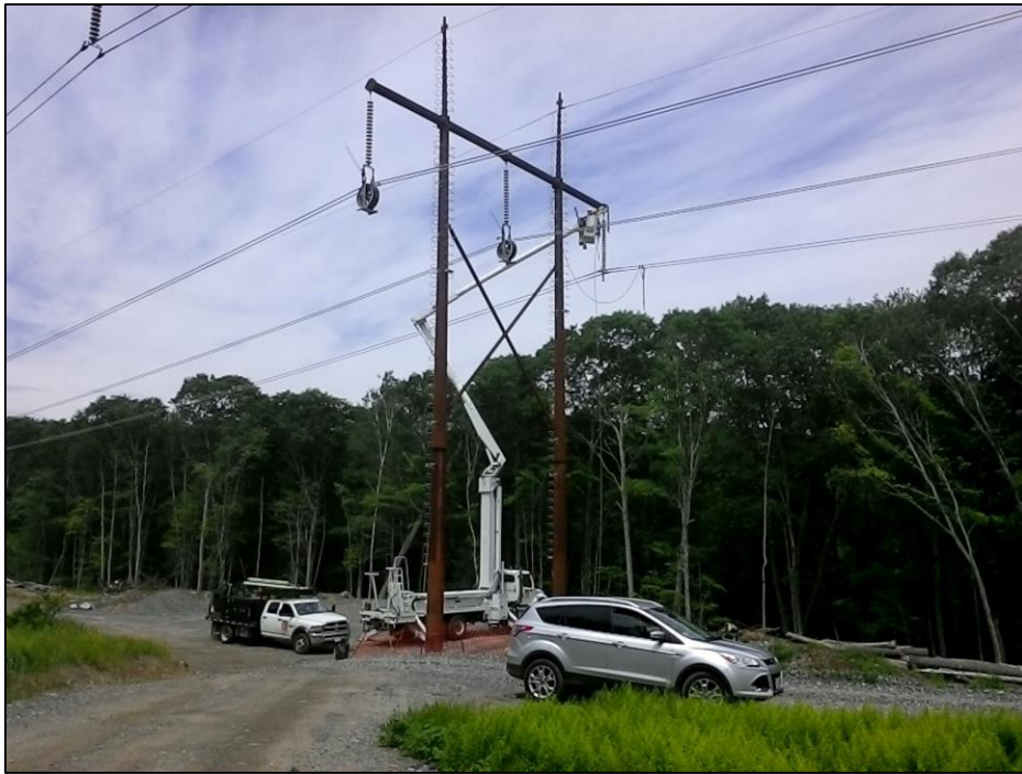
Photo #7: Conductor clipping at Str 313. (6/18)
