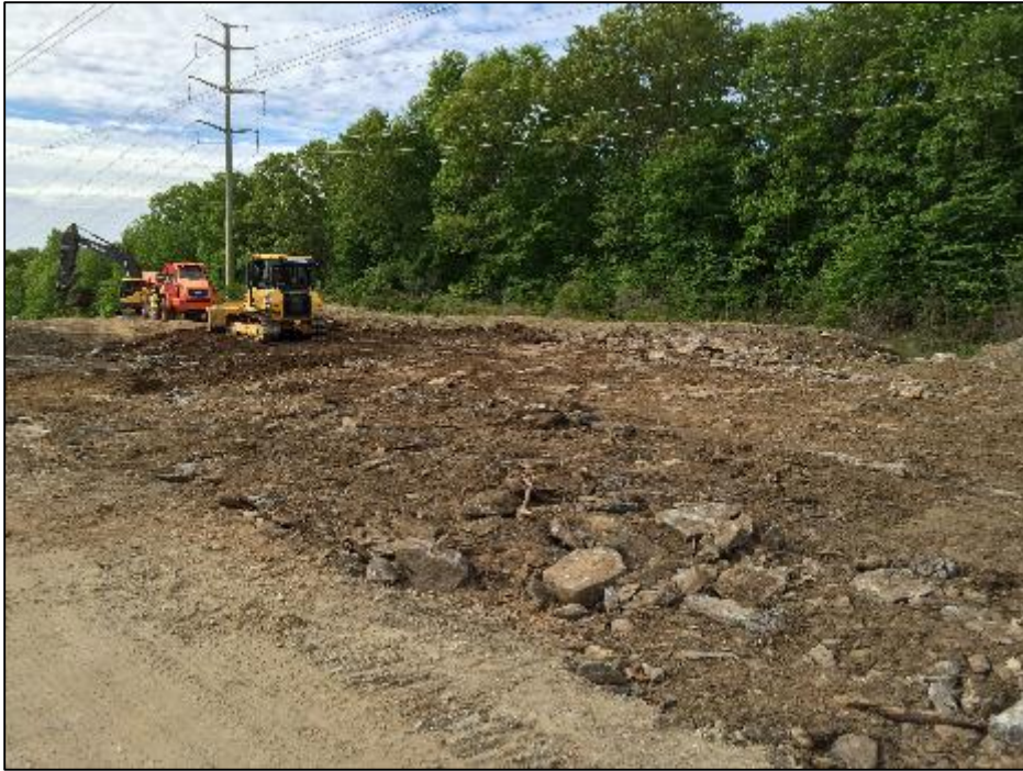
Photo #7: Removal of pulling pad between Str 16 and 17 as part of restoration. (5/21)
