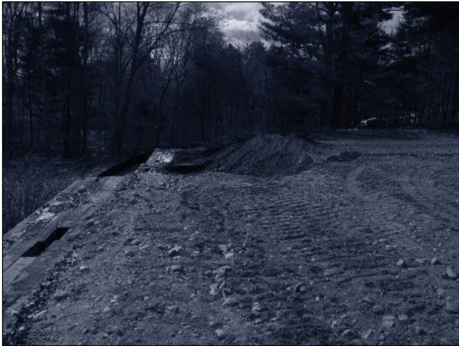
Photo #1: Removing temporary retaining wall as part of restoration operations at Str 80 pad. (4/30)
