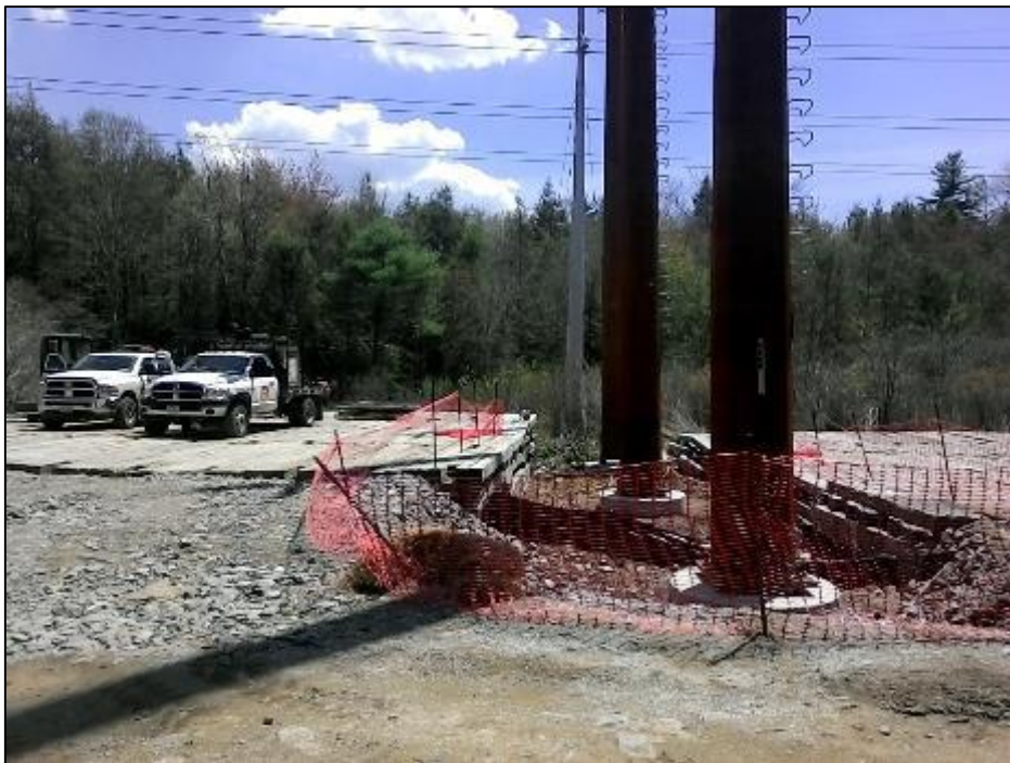
Photo #10: Grounding at Str 307.(5/8)
