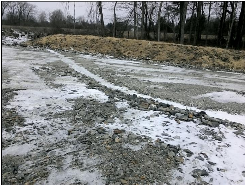
Photo #8: Waterbar installed across corner of pad upslope of wetland W20-188 entrance. (1/15)
