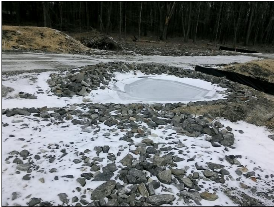
Photo #9: Sediment trap installed in accordance with BMP Manual and appears to be functioning correctly. (1/15)
