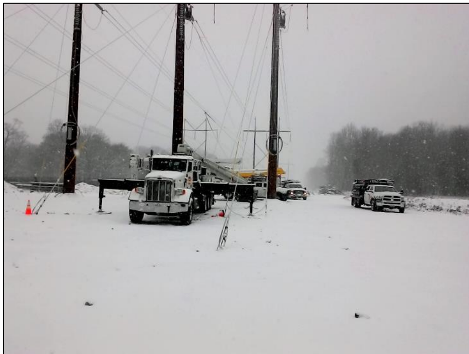
Photo #4: Line Crews preparing for conductor pull from Str 111-125 (Str 111 in view). (1/9)
