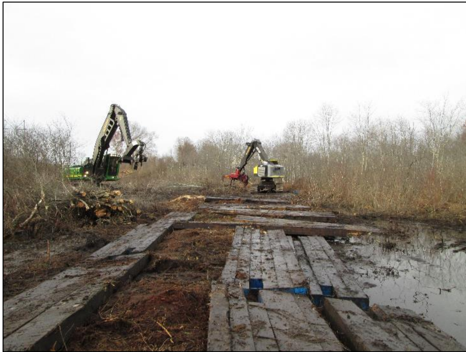
Photo #5: Clearing crew utilizing timber mats in wet areas to prevent unnecessary rutting between Str 298-299. (11/25)
