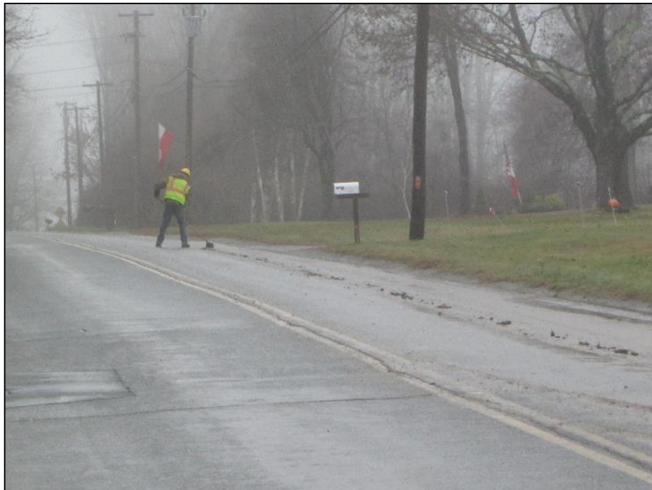
Photo #6: Observed sweeping of roadway after trucks leave construction site at Str 290. (12/3)
