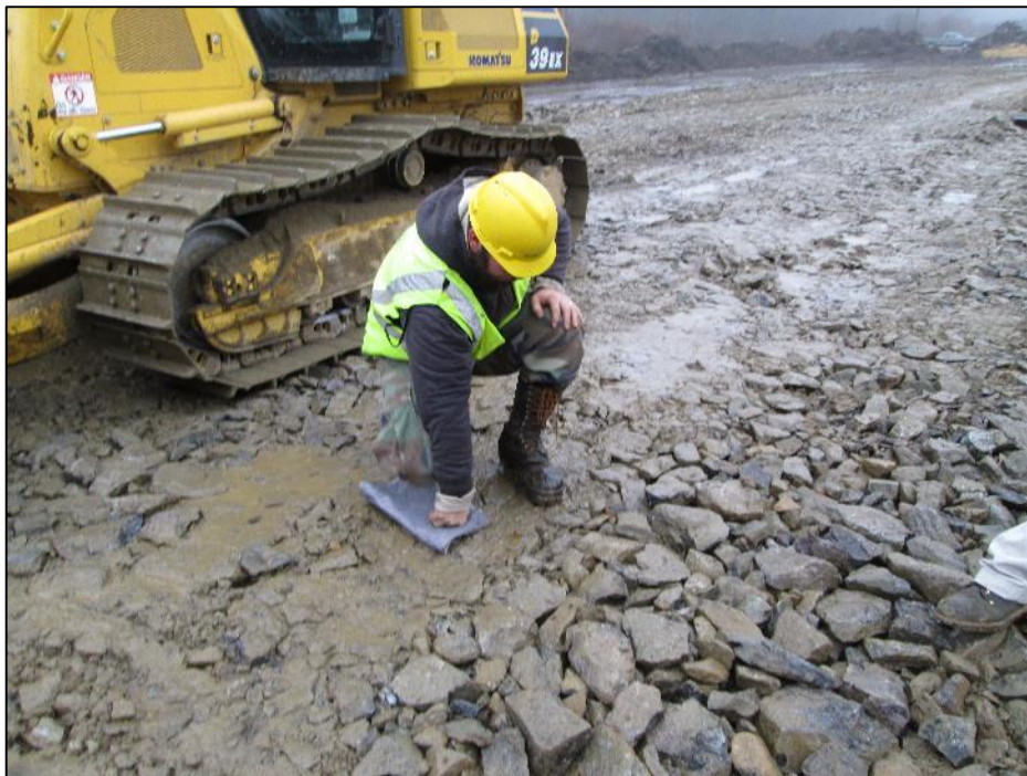
Photo #8: Northern crew immediately cleaned up drips with absorbent diapers at Str 290. (12/3)
