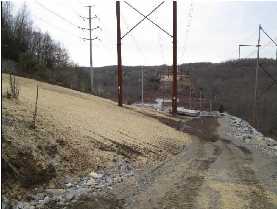
Photo #9: Erosion control of Str pad 22 restored to original grades and slopes. (11/25)
