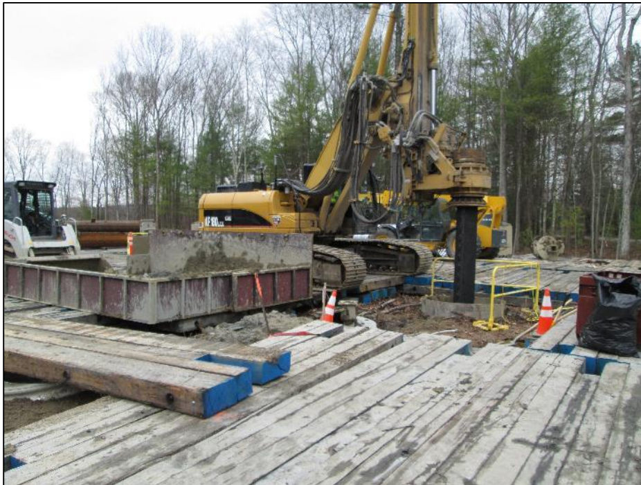
Photo #4: Spin off container and emergency spill protection under drilling machinery at Str 176. (11/25)
