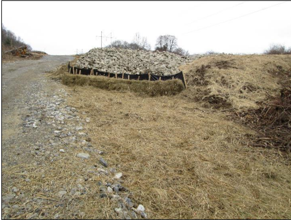
Photo #1: Observed plunge pool and hay bale reinforced silt fence at Str 284. (11/25)
