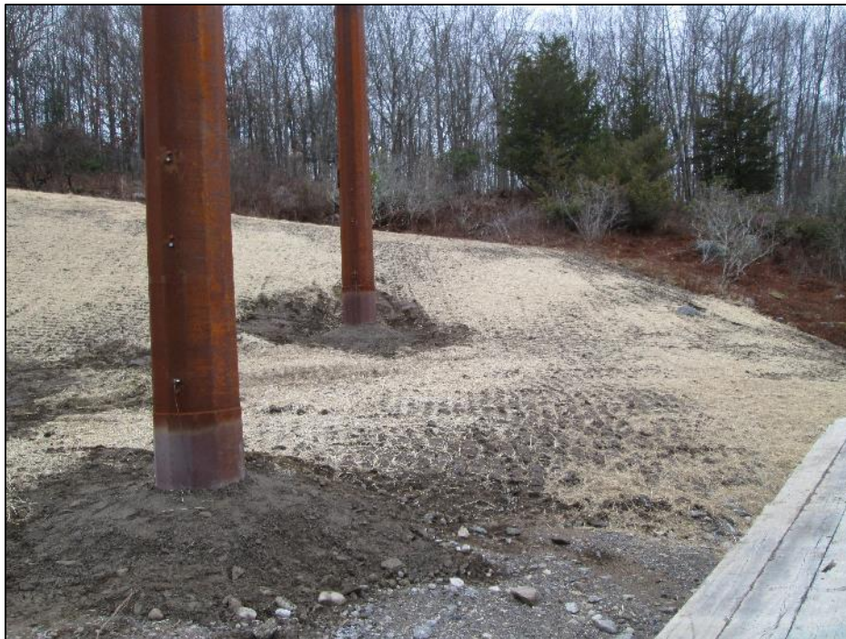
Photo #10: Erosion control of Str pad 22 restored to original grades and slopes. (11/25)
