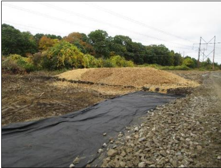
Photo #9: Striping of agricultural topsoil and installation of filter fabric at Str 227. (10/1)
