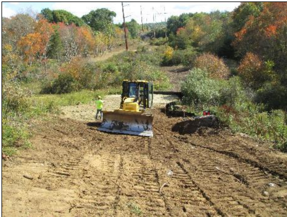
Photo #8: Spreading of hay over exposed topsoil and removal of fill up-line of Str 95.
