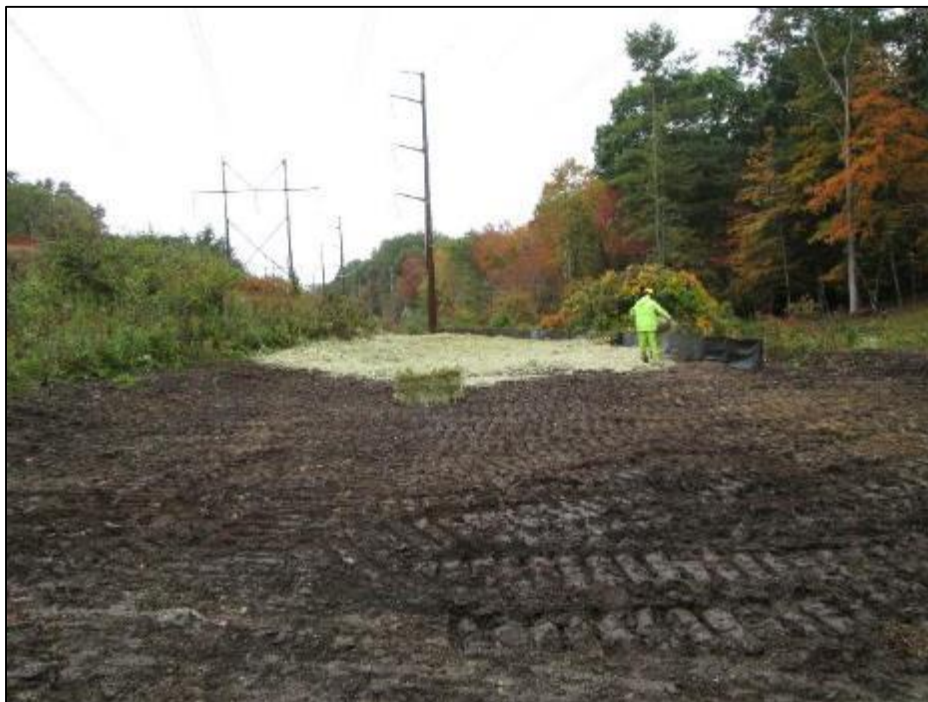
Photo #2: Spreading of hay and seed on exposed topsoil up-line of Str 99. (10/1)
