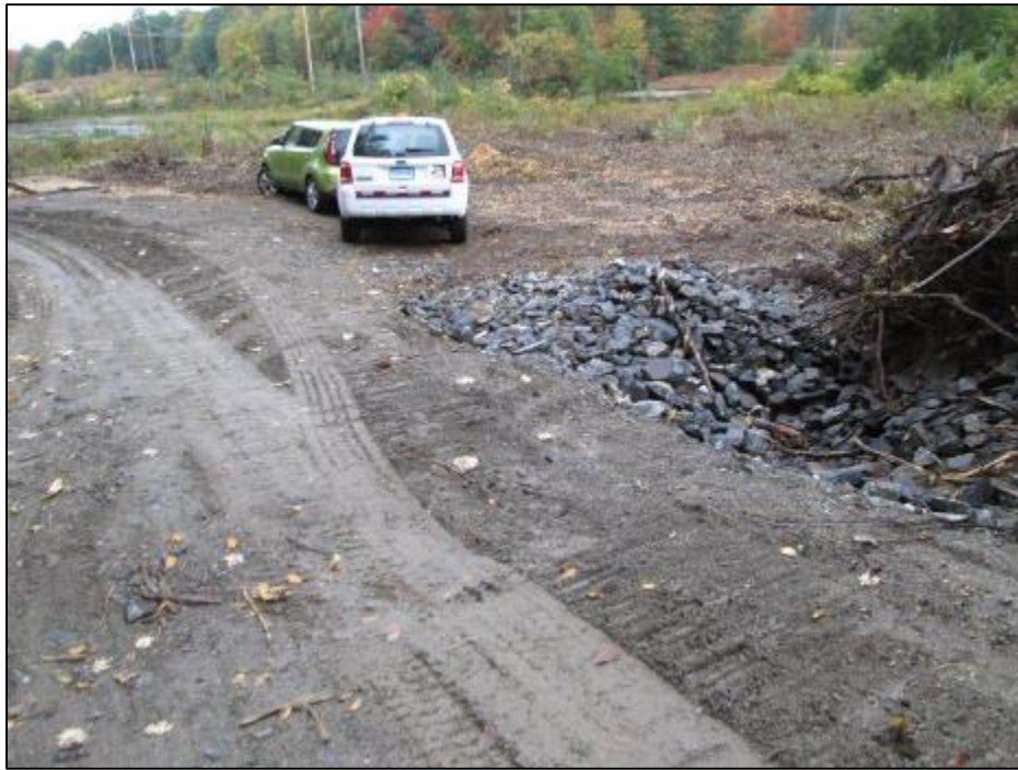
Photo #3: Plunge pool on edge of access road up-line of Str 202. (10/1)
