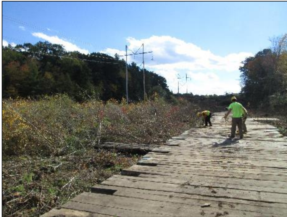
Photo #10: Connecting wetland mats with yellow rope in 100 year flood plain area between Str 206-207.
