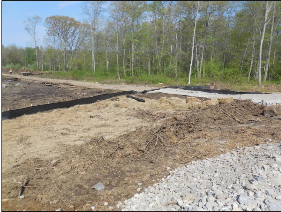
Photo #5: (5/14) Erosion control measures down-line of Str 29.
