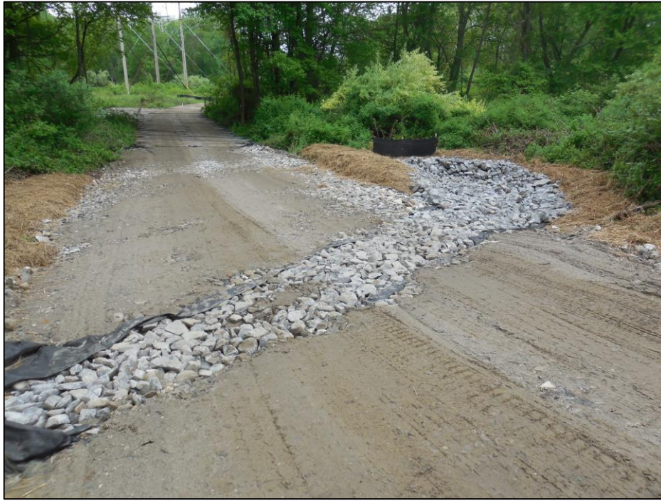
Photo #7: Erosion control measures on access road up-line of Str 55. Wetland mat installation visible in the background.
