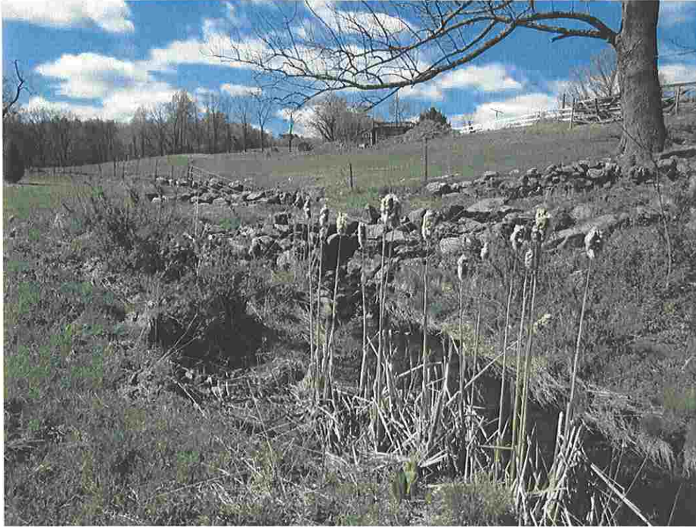
Photo 14: View of farm road crossing of Wetland 4, looking upstream (north) at culvert. (04/19/10)
