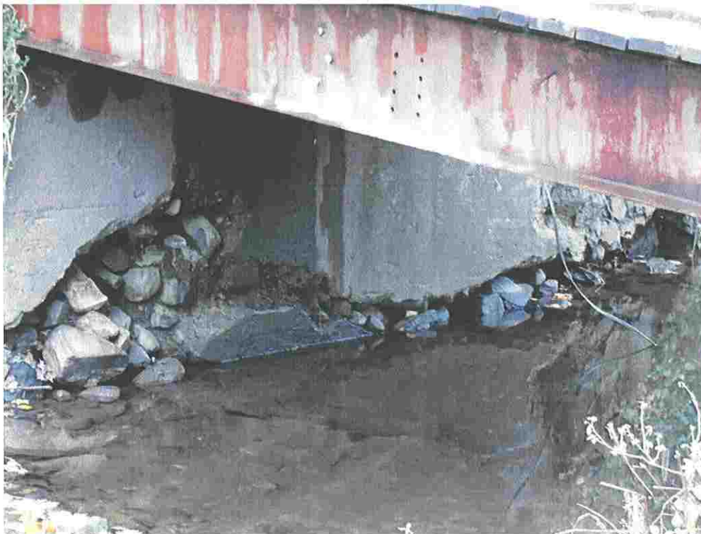
Photo 17: View of bridge abutment erosion, looking at west abutment. (10/05/10)
