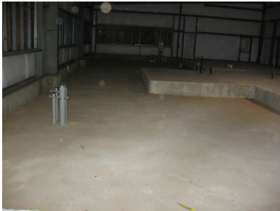
Control- Administration Building Interior showing lowered floor section with exposed pipes
