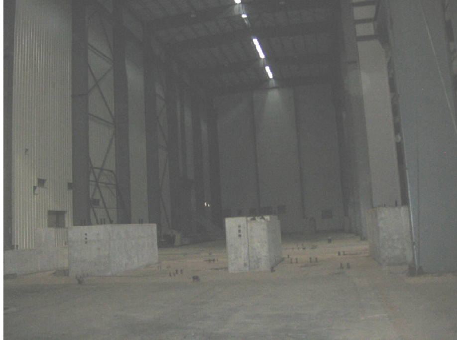
Power Plant Interior view
