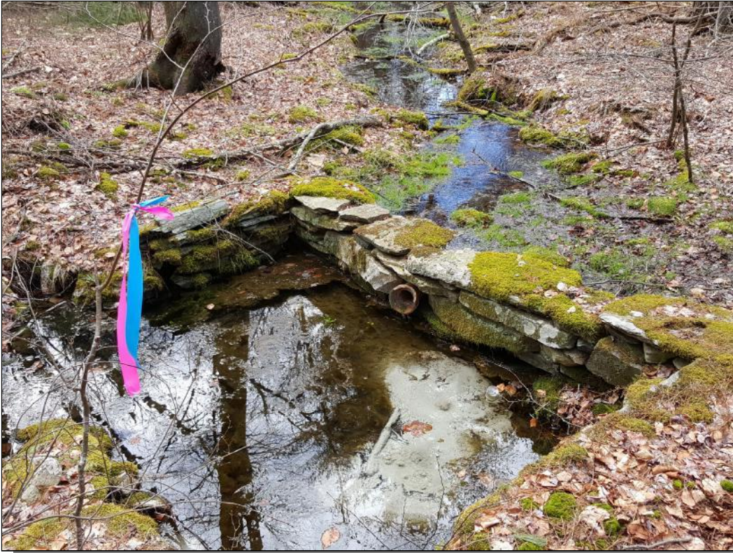
Photo A3-3: Wetland A3; cistern at spring at the headwaters of the wetland's watercourse; 3-18-16; facing westerly
