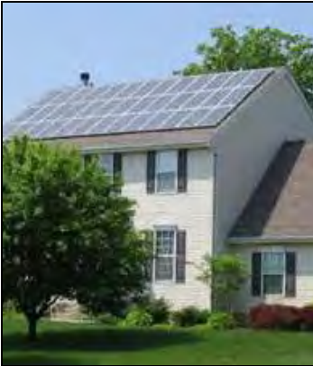
Residential Solar Installation
