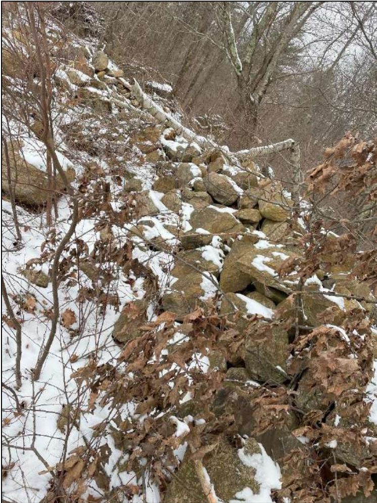
Photo 19. Overview of stone wall that extends past the project area. Photo taken facing north.
