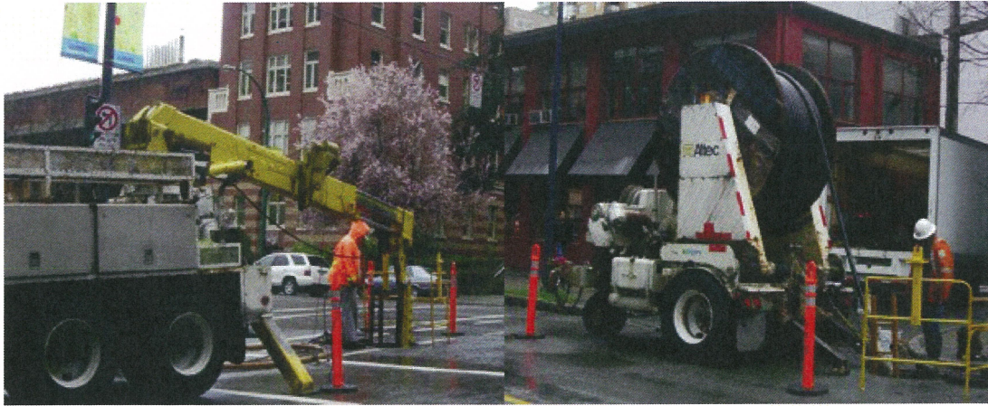
Figure 3. Underground cable upgrading program in a duct system, pulling (left) and cable feed (right). (Courtesy of BC Hydro/OCEI) [2]
