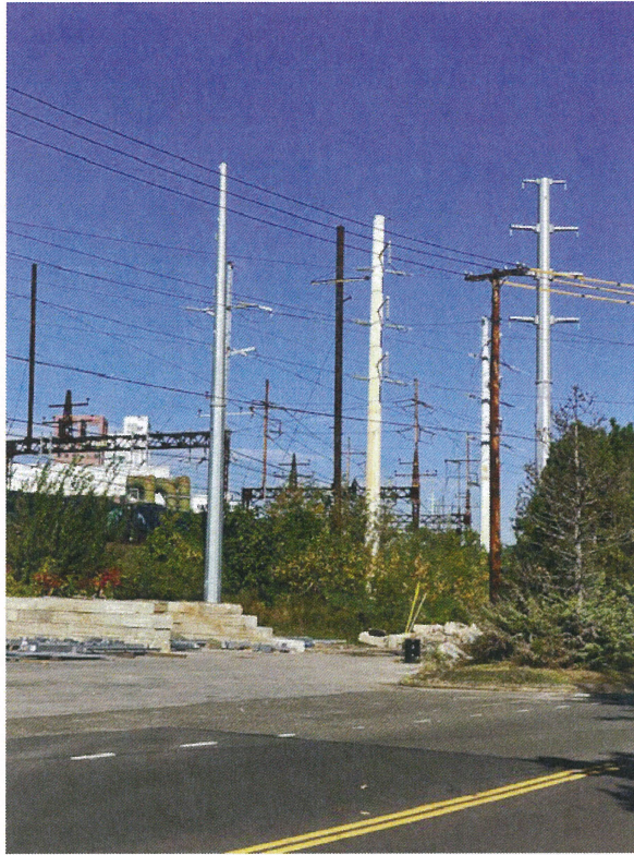
Figure 10, Overhead line congestion adjacent to Congress Substation.
