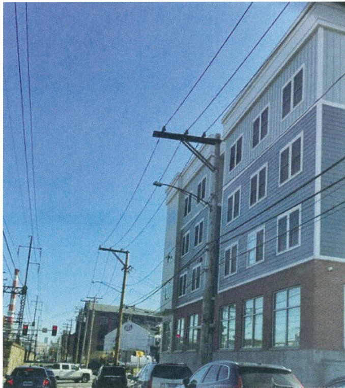
Figure 15. Dangerous OH line installation close to offices and apartments.
