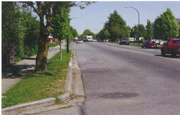
Figure 6. In-road installation of a 138 kV transmission cable. Only the manhole covers are visible. (OCEI)
