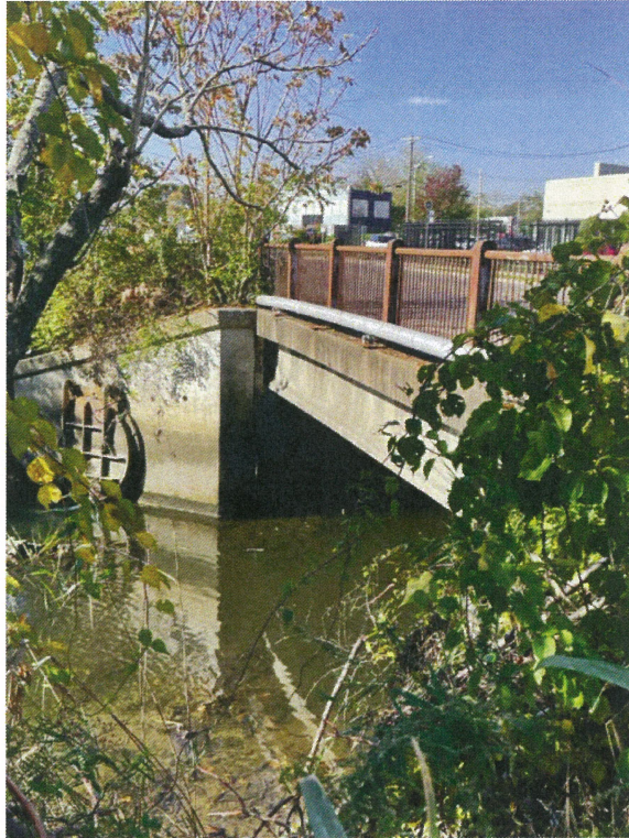
Figure 18. One of several river crossings at Mill River and Ash Creek. HDD, or support pipes attached to the bridge structure may be used.
