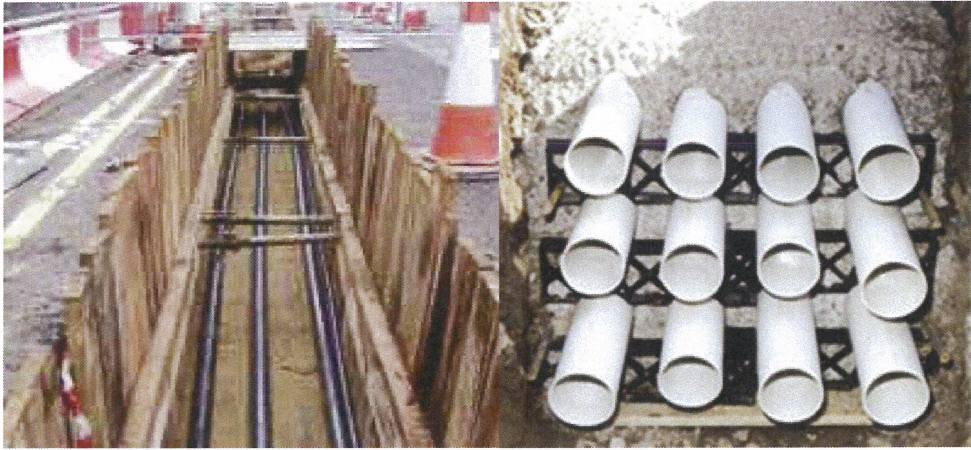
Figure 1. Trench design, direct buried flat configuration (left) and duct bank (right). (Courtesy Southwire) [2]
