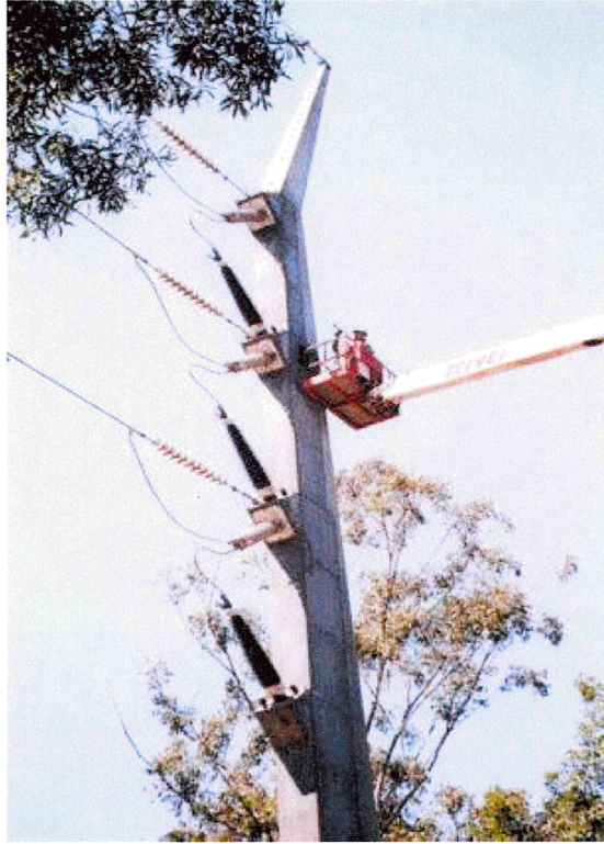
Figure 5. 110 kV single circuit vertical transition tower from OH to UG with well positioned surge arresters. (Courtesy of Powerlink) [2]
