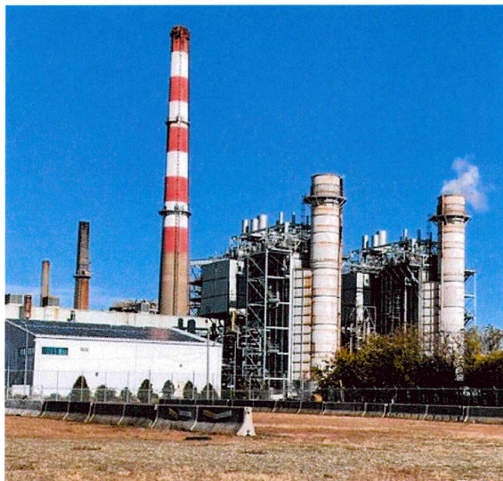
Figure 9. Bridgeport generation plant.
