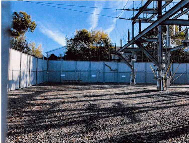
Figure 12. Ash Creek Substation yard with ample room for UG cable terminations.
