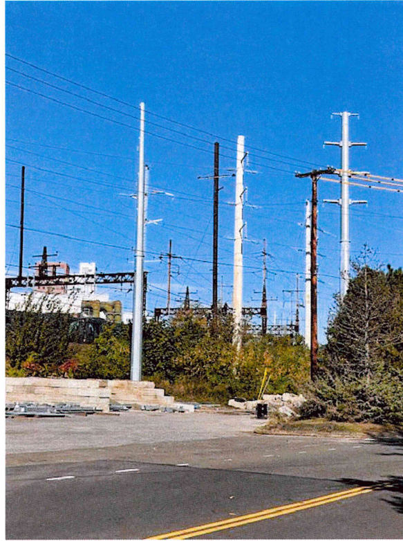
Figure 10, Overhead line congestion adjacent to Congress Substation.
