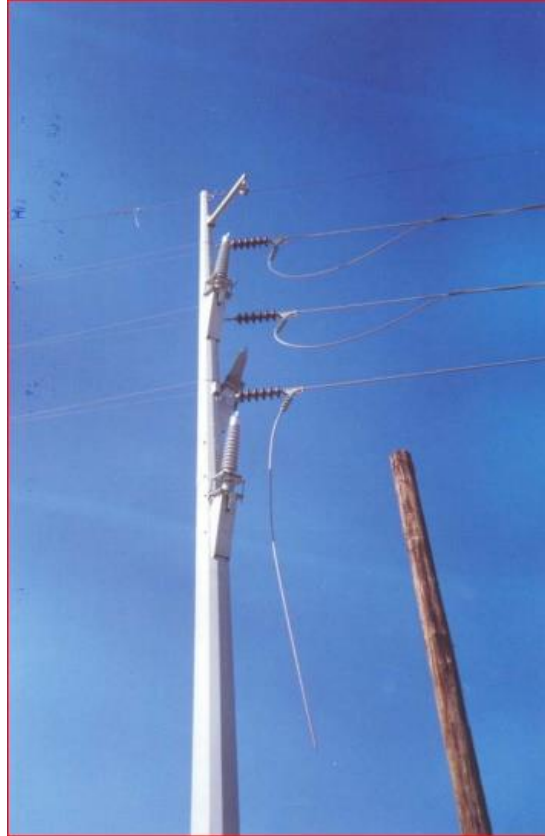
Figure 7. Transition of one circuit from OHTL to underground cables (Ref. CIGRE TB-250)
