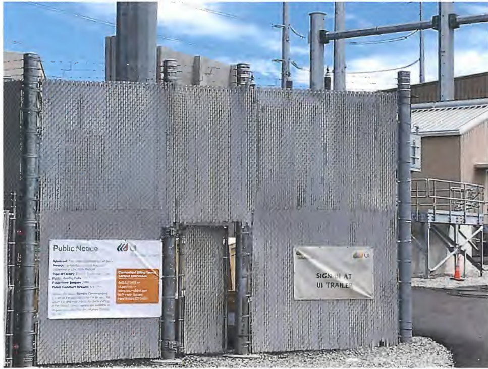
UI's Pequonnock Substation at 1 Kiefer Street, Bridgeport, CT
