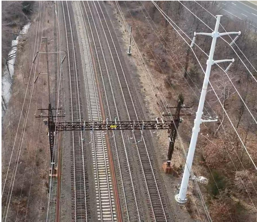
Figure 1-3: Representative UI Bonnets on Southern Railroad Catenary Structure and Line 1130 on Monopoles on North Side of Railroad Tracks (Town of Fairfield; View to the West)
