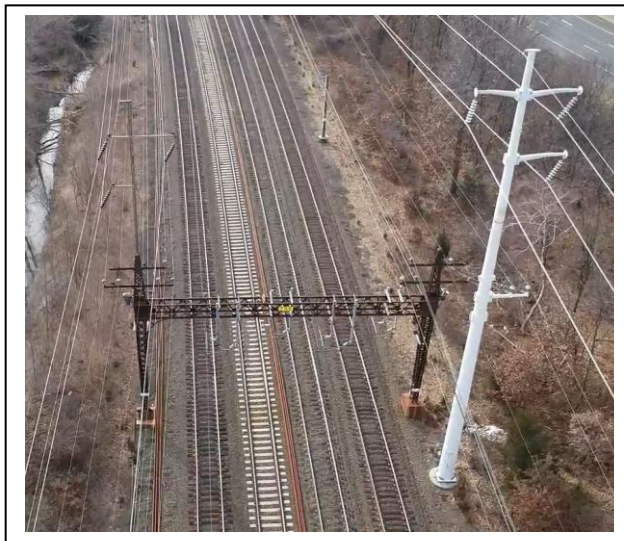
Figure 2: View of UI Infrastructure on Southern Catenary Structure and 1130 Line Monopole North of MNR Tracks (Fairfield)
