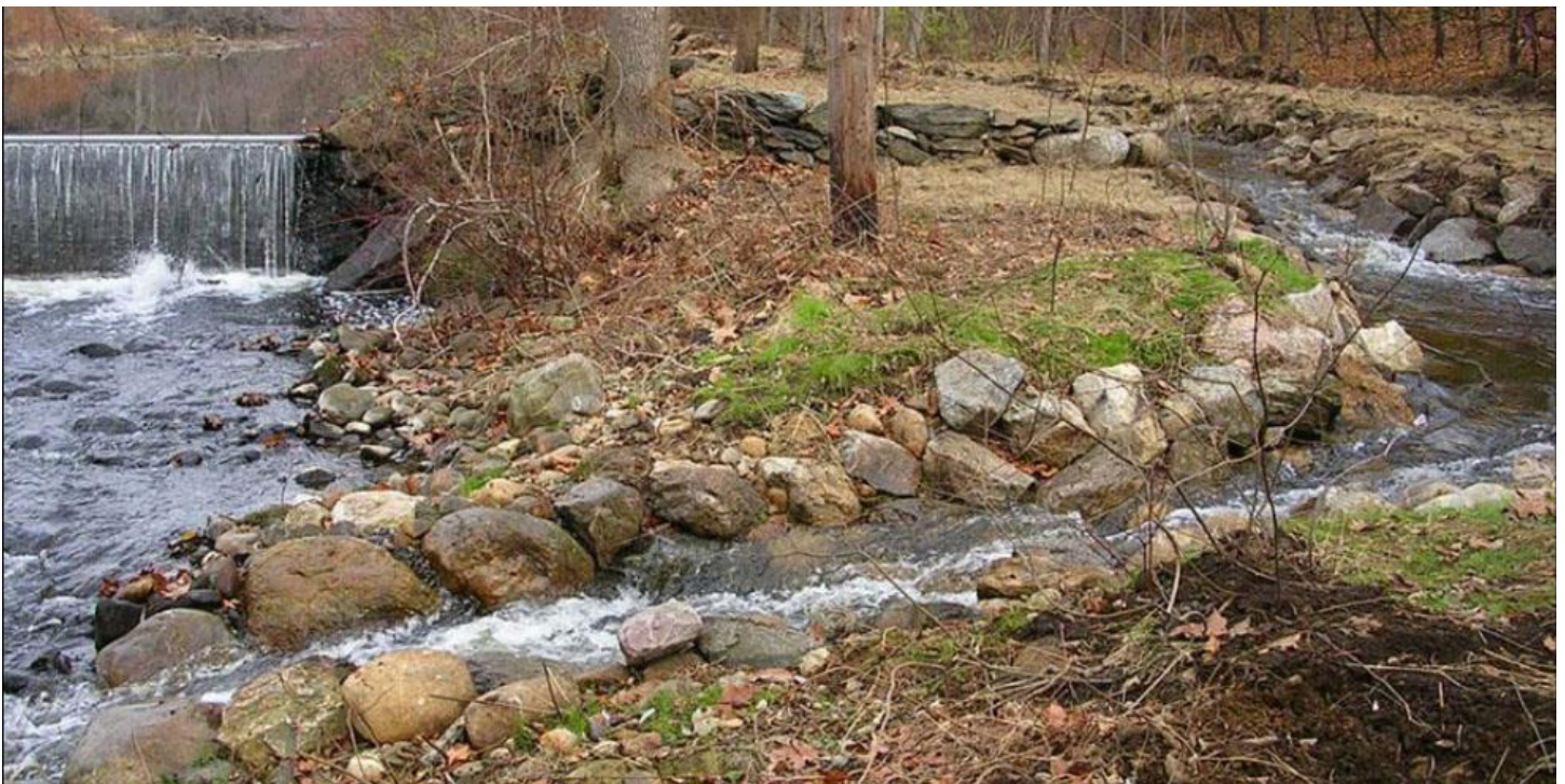
The Cannondale Fish Bypass is part of an ongoing effort to restore migratory fish habitat on the Norwalk River Photo Credit: Milone & MacBroom, Inc.
