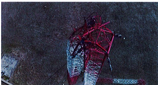
Tornado damages tower array Moore, OK, March 25, 2015 http://qrznow.com/tornado-damage-to-
