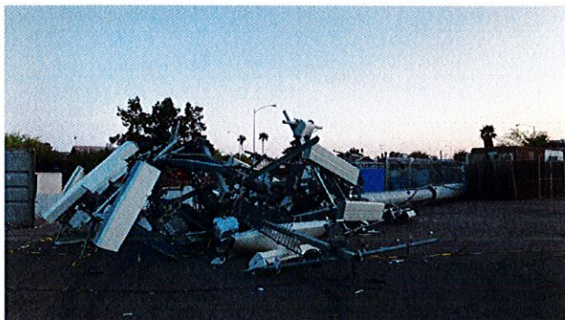
Cell tower collapses feet from homes and businesses due to high winds Las Vegas, NV, Apr. 25, 2022
