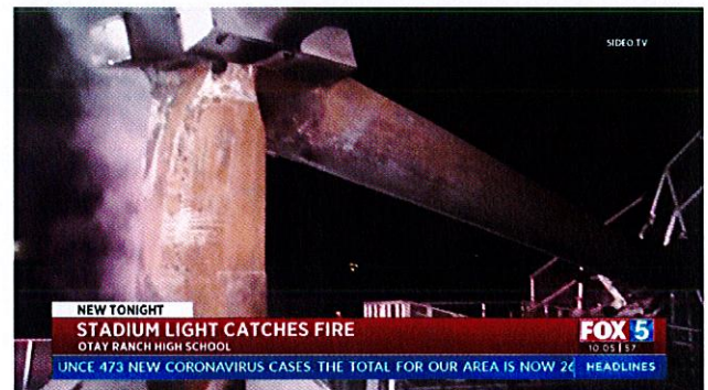
A light pole holding cellular antennas at Otay Ranch High School caught fire,
