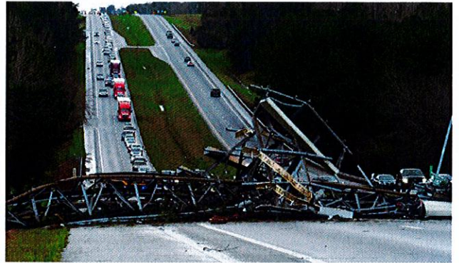
Cell tower felled by tornado across U.S. Route 280. Smiths Station, Lee County, AL, March 3, 2019 https://www.nytimes.com/2019/03/03/us/tornado-alabama-georgia-deaths.html Photo credit: Mike Haskey/Ledger-Enquirer, via Associated Press
