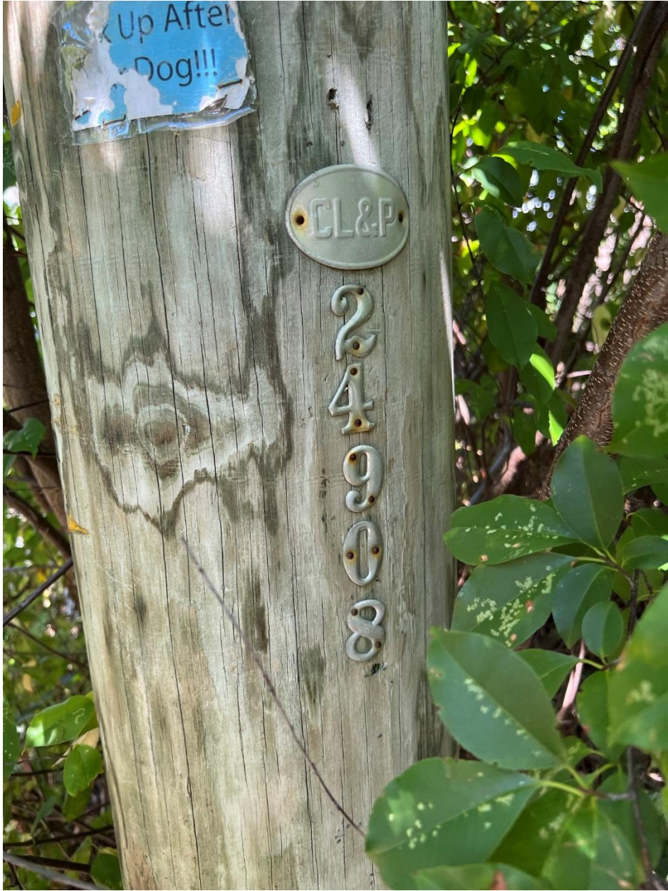
Existing Utility Pole that would be used to provide Power and Telco to Site
