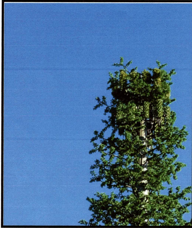
120' tall stealth stealth monopine by Homeland Towers at the Pehquenakonck County Club, North Salem, NY. Verizon and AT&T antennas concealed within branches.
