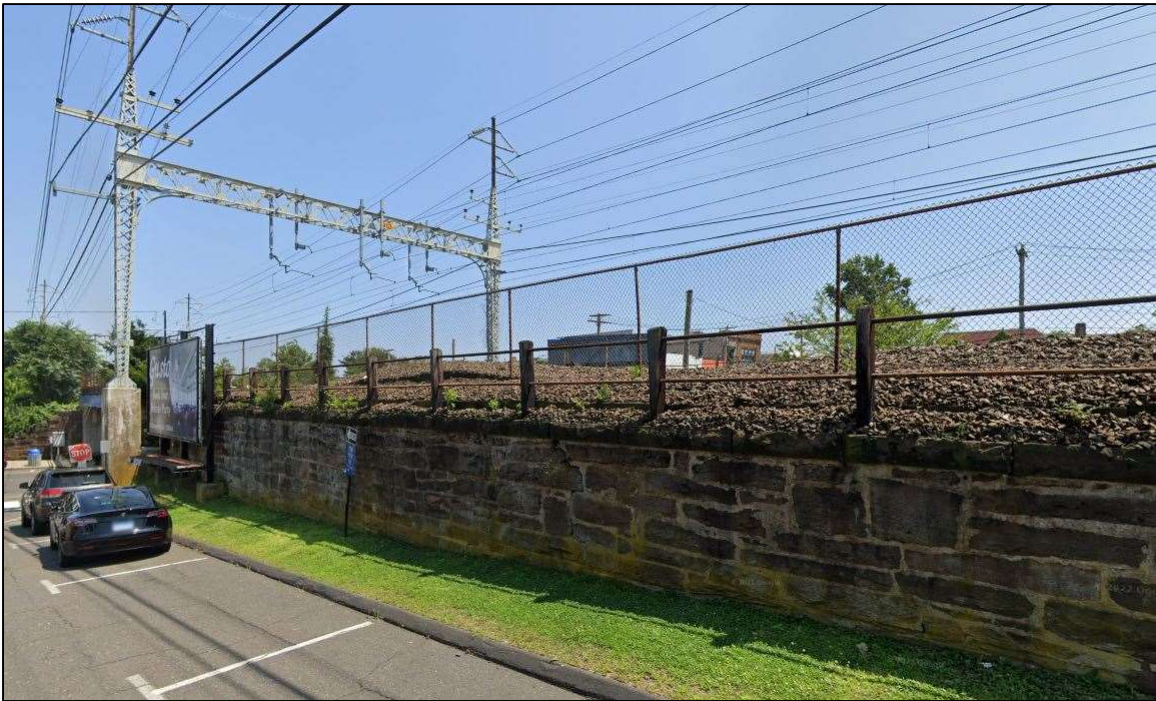
21 View of NRHP-eligible rail line with historic stone retaining walls along Railroad Avenue west of 22 River Street, camera facing southeast (Google Street view photo).
