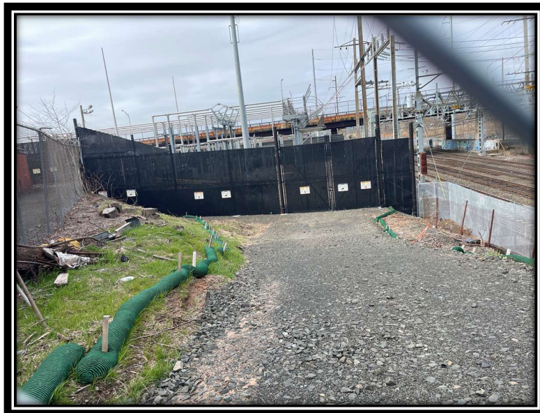
Photo 2: Permanent road installation off Grant Street and into the West River Substation. Completed with erosion controls, mulching, and seeding.
