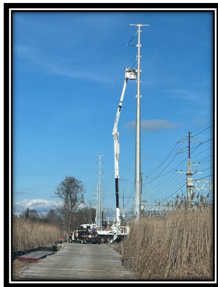
Photo 4 : Overhead work along temporary access road, west side of the West River.
