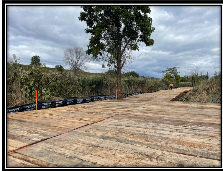
Photo 3: Matting through wetland area, located on western side of the West River.
