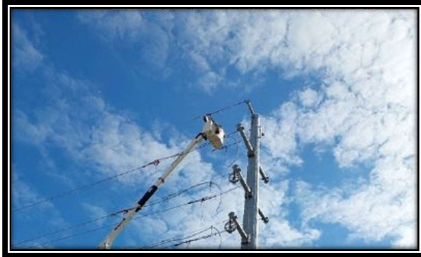
Photo 3: Typical overhead utility work.
