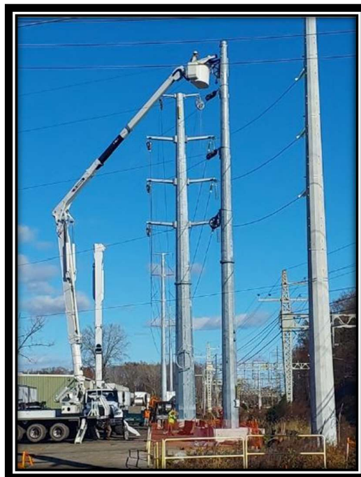
Photo 4 : Typical overhead utility work
