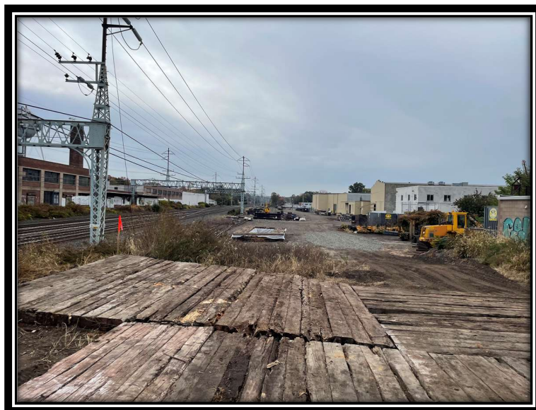
Photo 10: Work pad associated with P1038N, facing west, and overlooking MNR railyard. Small concrete washout located in the distance.
