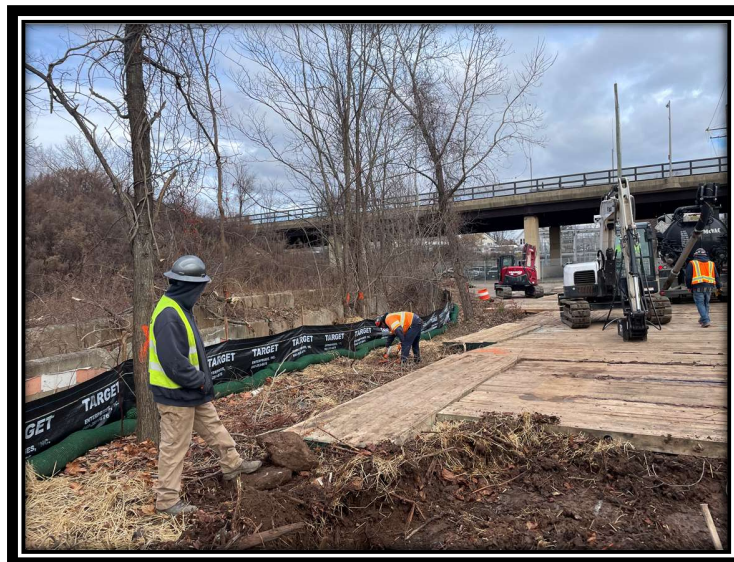
Photo 16: Work pad construction at P1049N, located on the east side of the West River. Trees marked in orange were cut flush to the ground. Minor clearing within work pad area (listed as a minor deviation).
