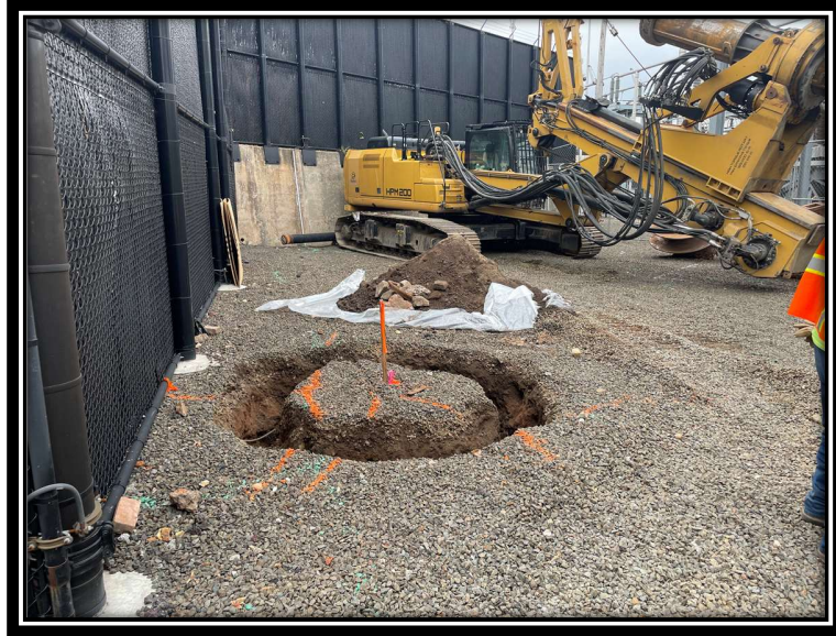
Photo 1: Typical soft dig, mid-process. Photo taken at P1050NS and within the West River Substation.
