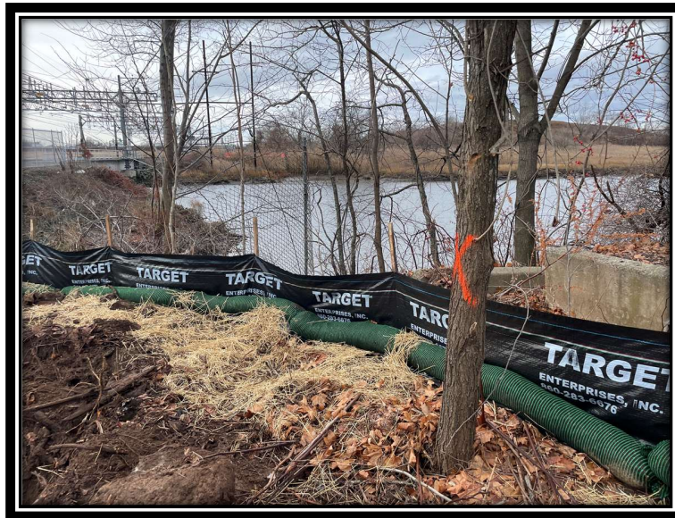
Photo 17: Extent of work area associated with P1049N, facing east and across the West River. Photo shows exclusionary/redundant silt fencing, and temporary seeding/straw mulching. Tree marked orange cut flush to the ground (listed as a minor deviation).
