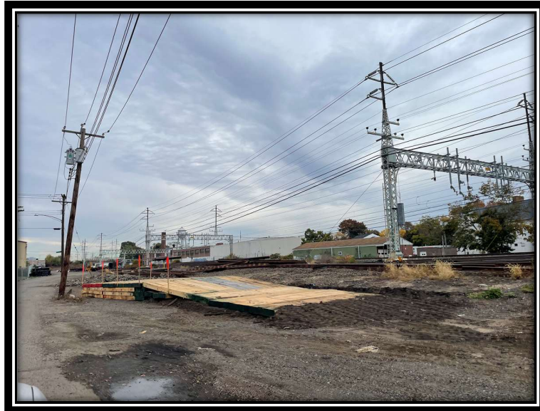
Photo 9: Work pad located within MNR rail yard and off Washington Ave. This work pad is associated with P1035N.
