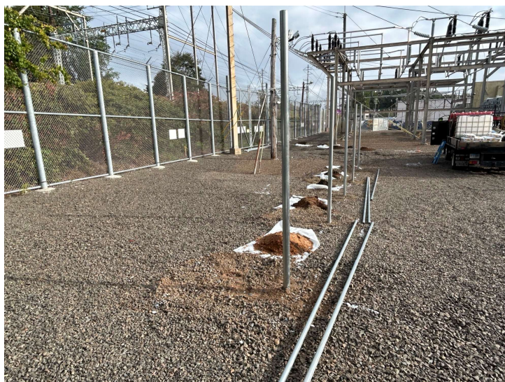
Photo 2: Temporary fencing inside Elmwest Substation, used to gain access to install structures P1029WNS and P1029SS.
