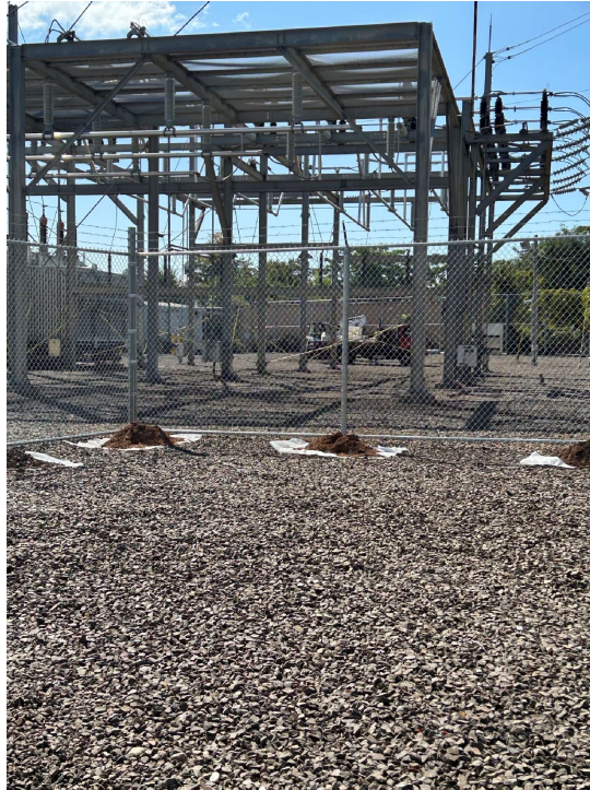
Photo 1: Temporary fencing inside Elmwest Substation, used to gain access to install structure P1029ES.
