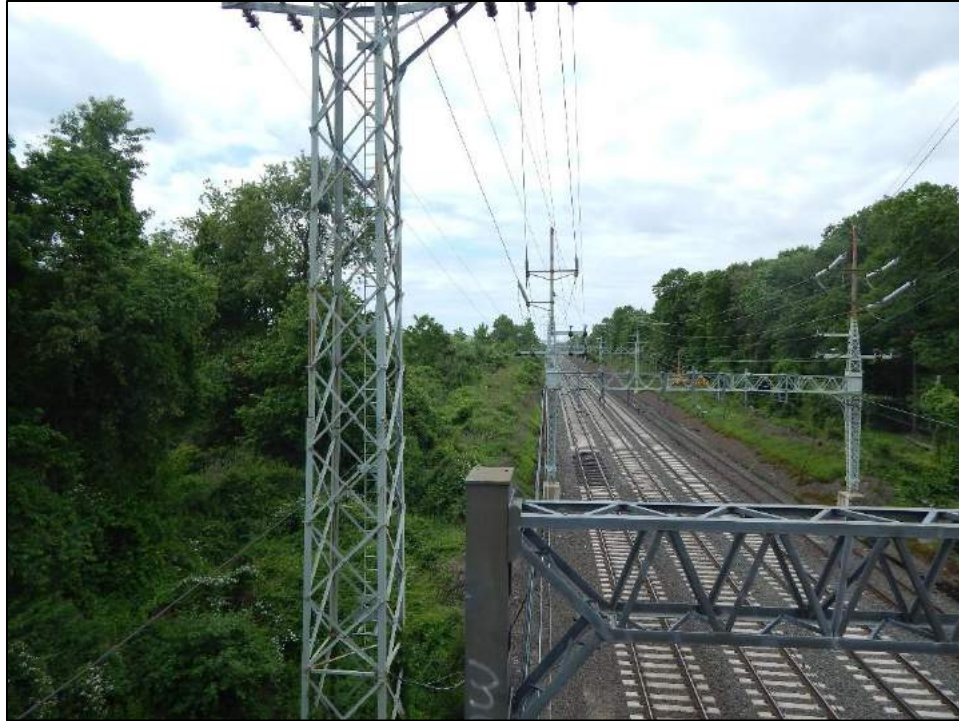
Figure 32. Overview photo of existing CT DOT corridor looking southwest from the Allings Crossing Road Bridge crossing in West Haven.
