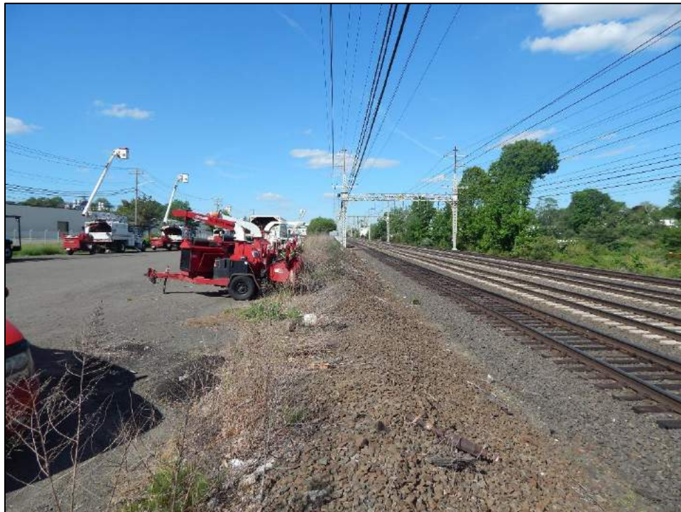
Figure 31. Overview photo looking northeast showing proposed work/pulling pad and proposed access road along the existing CT DOT corridor near Heffernan Drive in West Haven.
