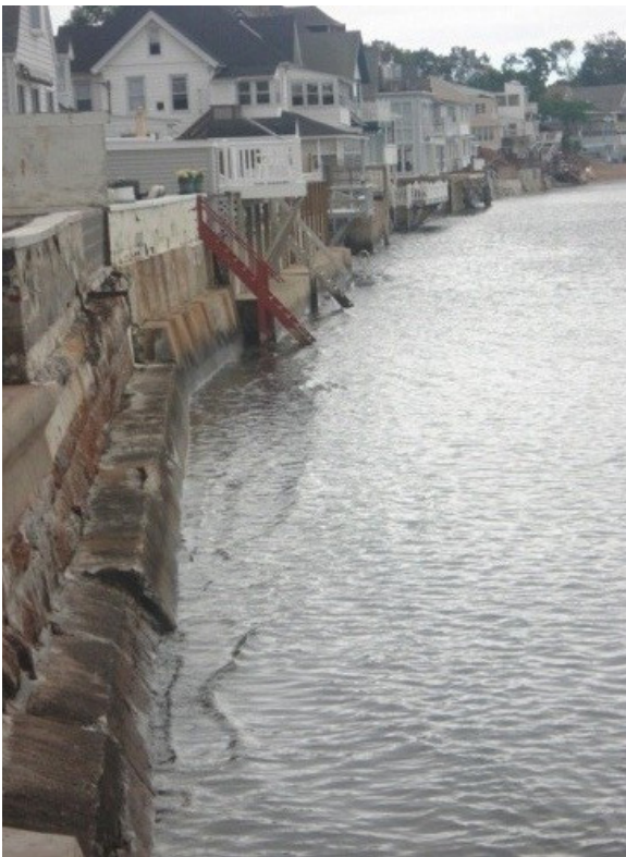
View of properties at risk at Pardee seawall in Morris Cove neighborhood.
