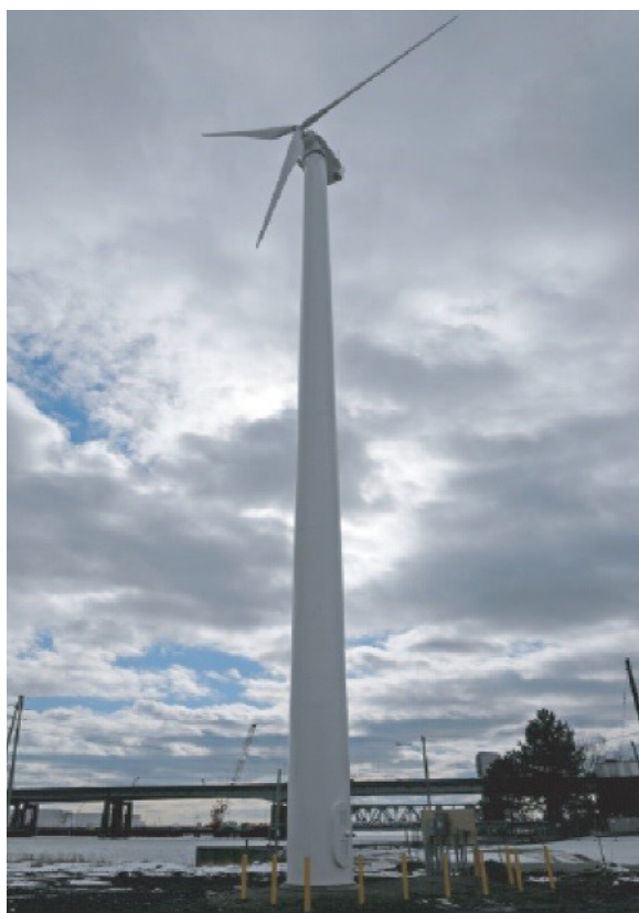
Phoenix Press on James Street installed a 100 kW wind turbine to provide a third of its electricity needs in 2010.
