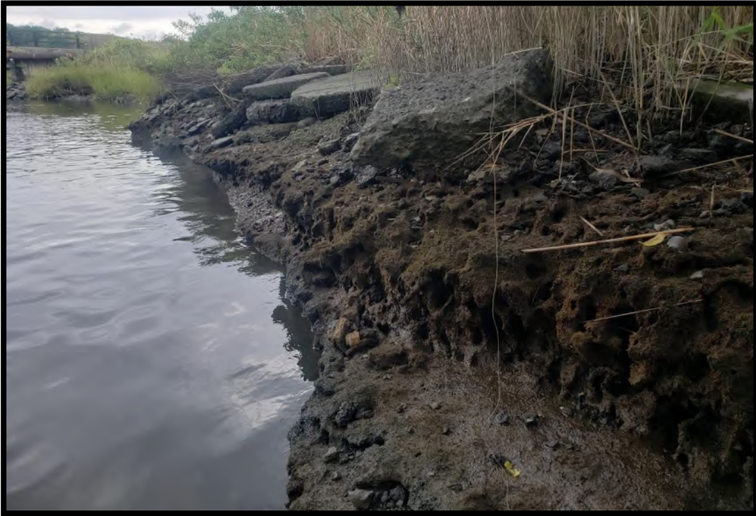
Photo 45: Asphalt dominated shoreline, with some muddy bank areas. Note riprap shore in background. Photo taken looking south. 9/16/2021.
