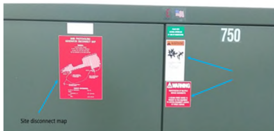
Typical Transformer Signage/ NFPA
