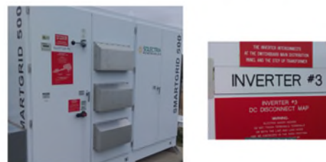
Typical Inverter Signage /NFPA
