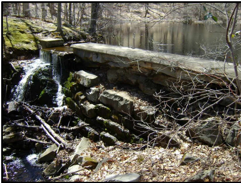
Photo of Putnam Memorial Park Pond Dam in Redding
