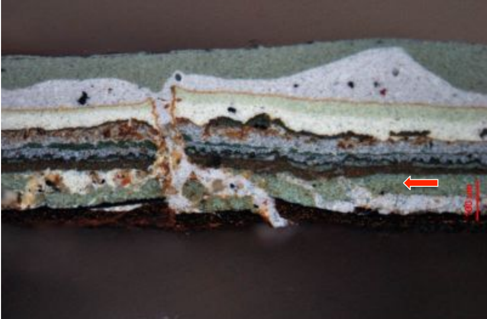
Figure B9a: Cross Section, Sample G, spandrel column, brightfield, 100x magnification. Red arrow indicates the location of the original, medium green finish.
