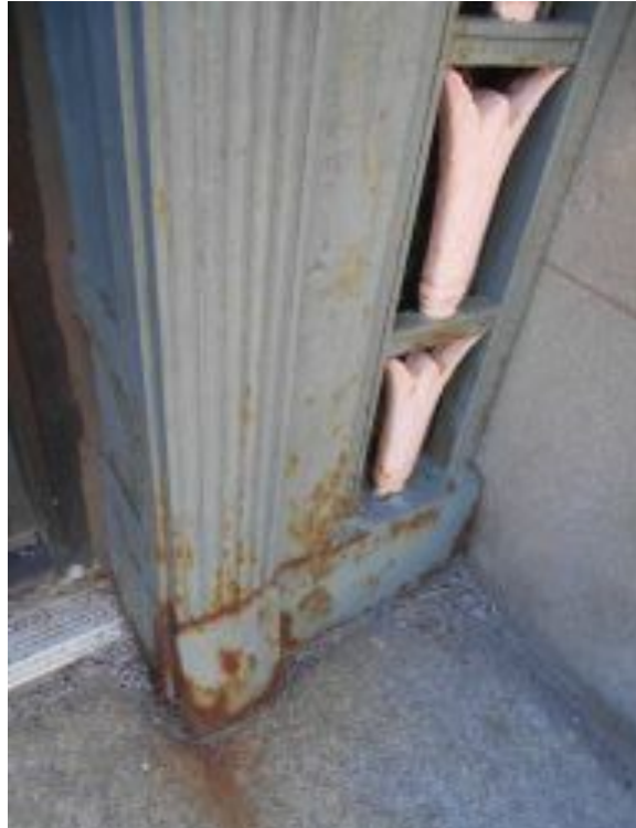
Figure A3. North elevation contemporary detail of west door showing corroded metal substrate condition.
