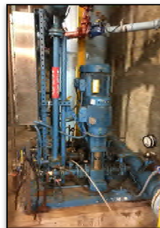
Plant Water System
