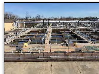
Primary Settling Tanks
