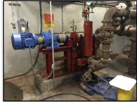
Primary Sludge Pumps
