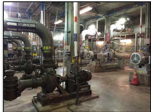
Return Sludge Pumps
