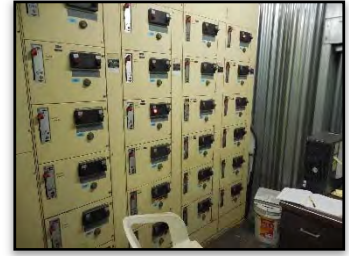
Compost Building MCCs
