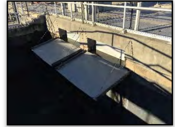
Zone A Aeration
