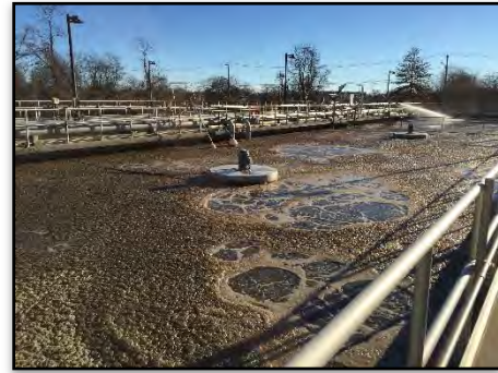
Zone B Aeration Tanks
