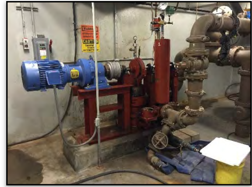
Primary sludge pump
