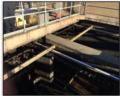
Primary Settling Tanks
