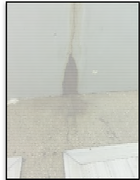
Subgrade Wall Leaks
