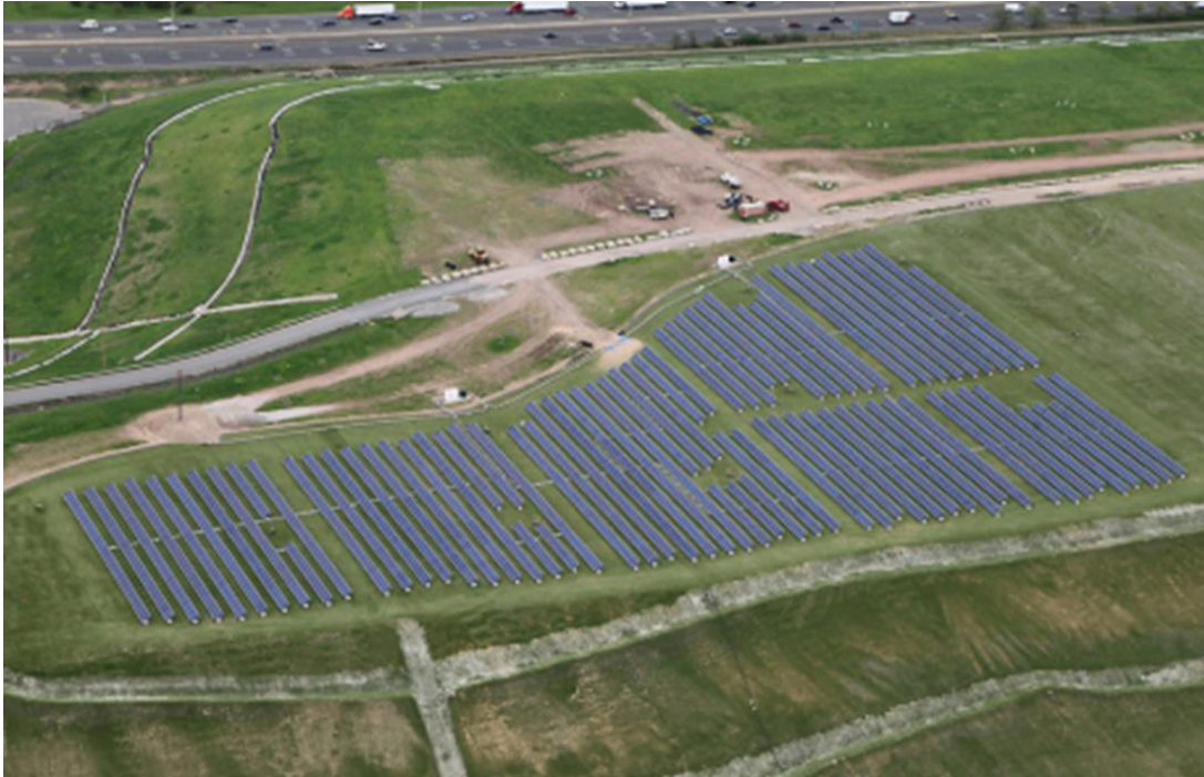
August 2014: the Hartford Landfill 1 MW solar array starts production
