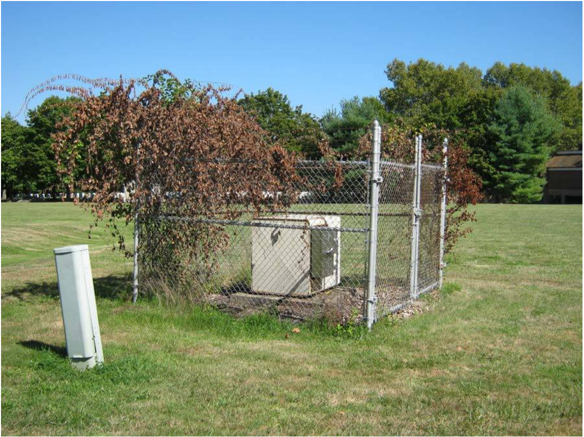
Photograph 5: Facing northeast to an above-ground electrical box in the Cemetery Expansion Area of Potential Effect (APE) that connects to underground electrical lines from Holmes Drive to the west.
