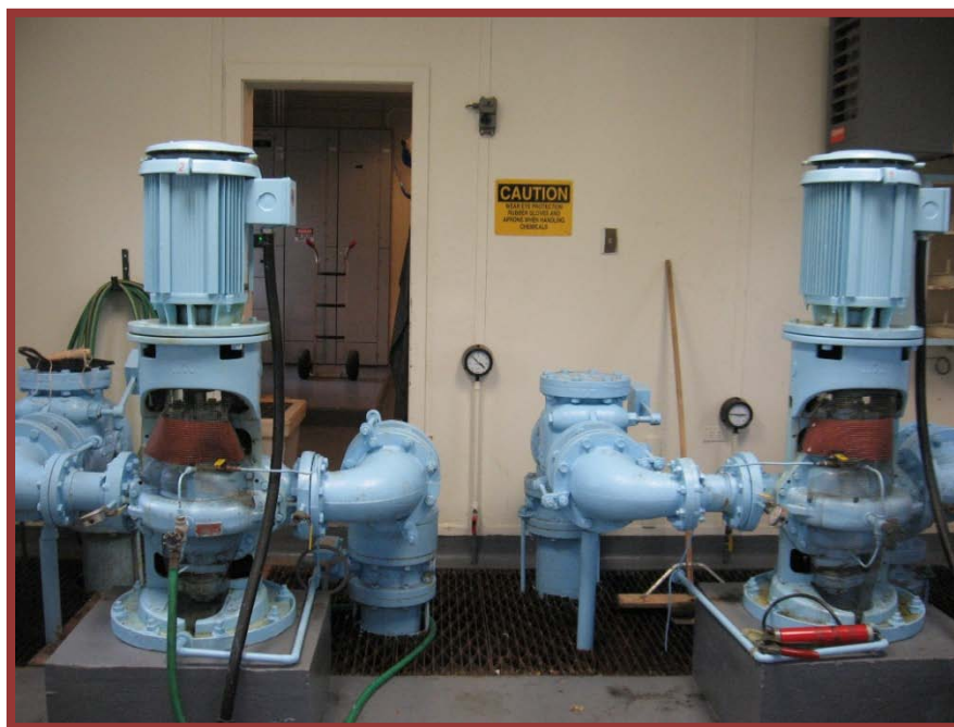
Photo 4 - View of pump units in Room 1 of Pump Station.
