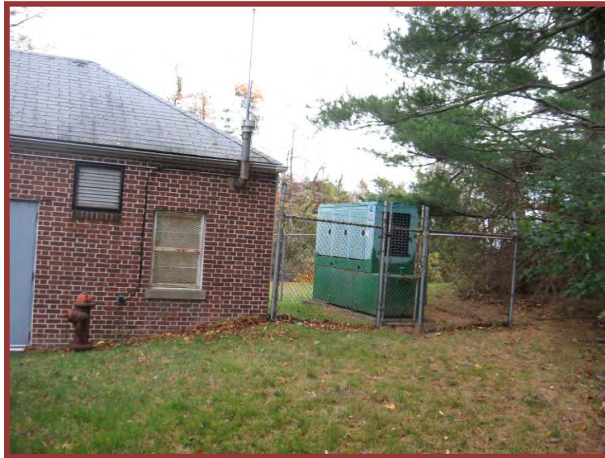
Photo 3 - View of fenced area where generator is located, facing southeast.
