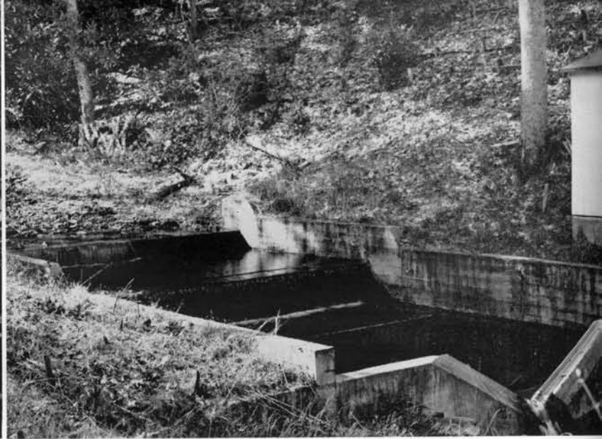
Thirty of these stream gauges, operated since 1934 by the Forest Service at the Coweeta Hydrologic Laboratory, enable scientists to measure water flow.
